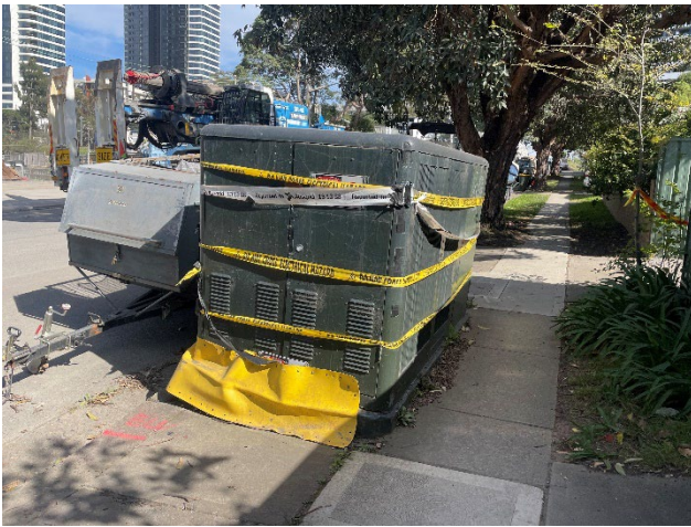
Figure 25 – View of the electricity substation present on Llewellyn Street.
