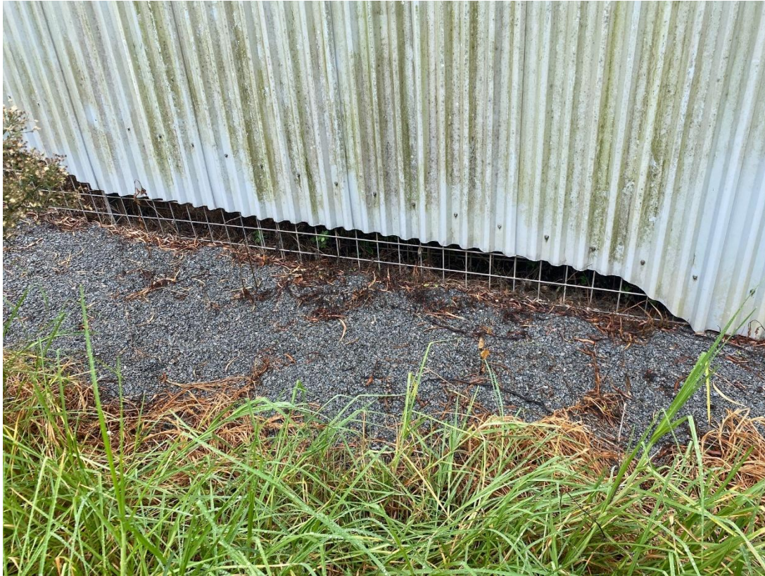
Photograph 4.2 Example of gaps at the base of the fence, in the green space
