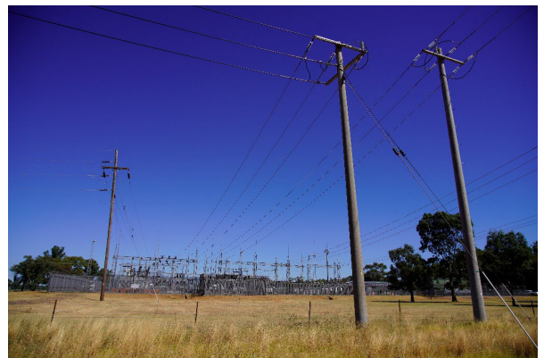
FIGURE 5-2 EXISTING YANCO TRANSGRID SUBSTATION
