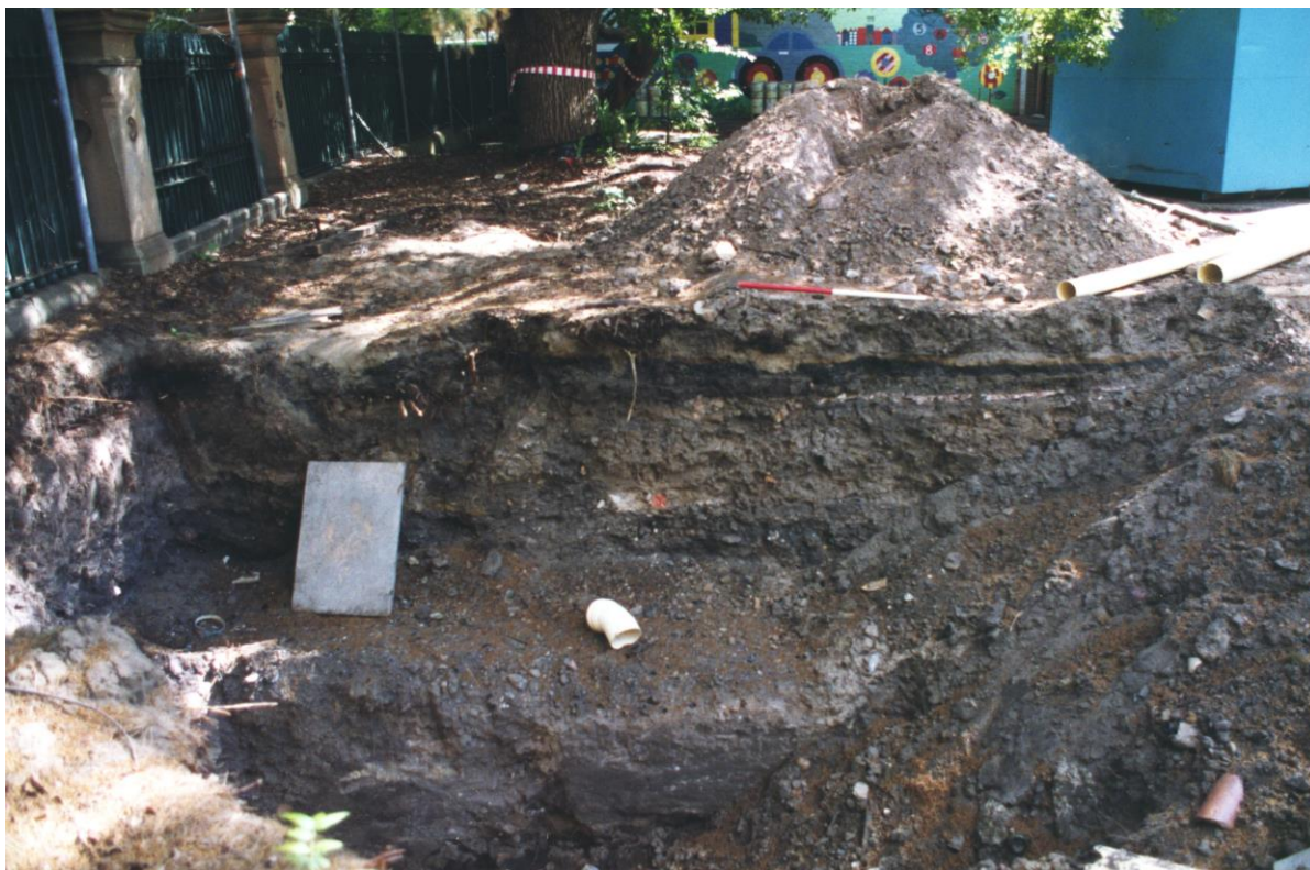
Figure 4.12: South-facing section of gas main trench, Trench 1. Photo taken looking north, BLKF 2.5, Scale 1m.
