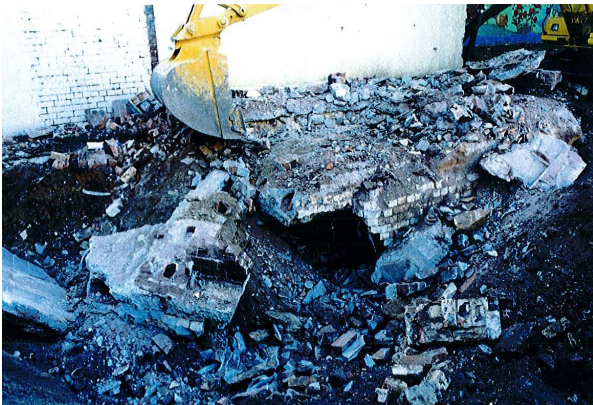
Figure 4.23: Extensive brick footings below the toilet block in the area of the new Childcare Centre. Photo taken looking north, BLKF 3.35.
