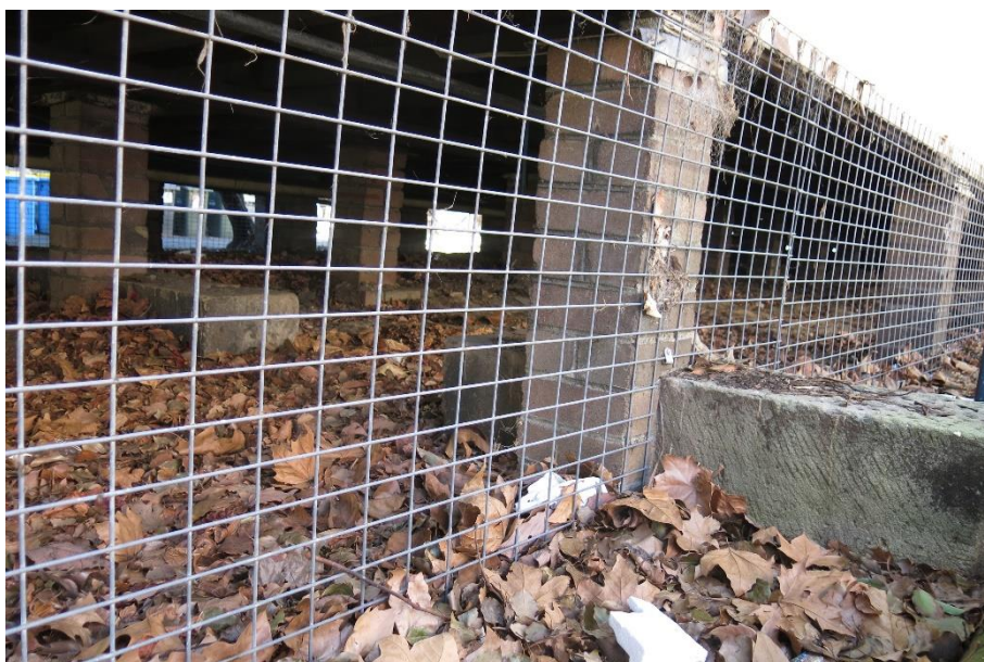
Figure 4.6: Detail showing sandstone blocks beneath timber building in southwest corner of site. Looking northeast.
