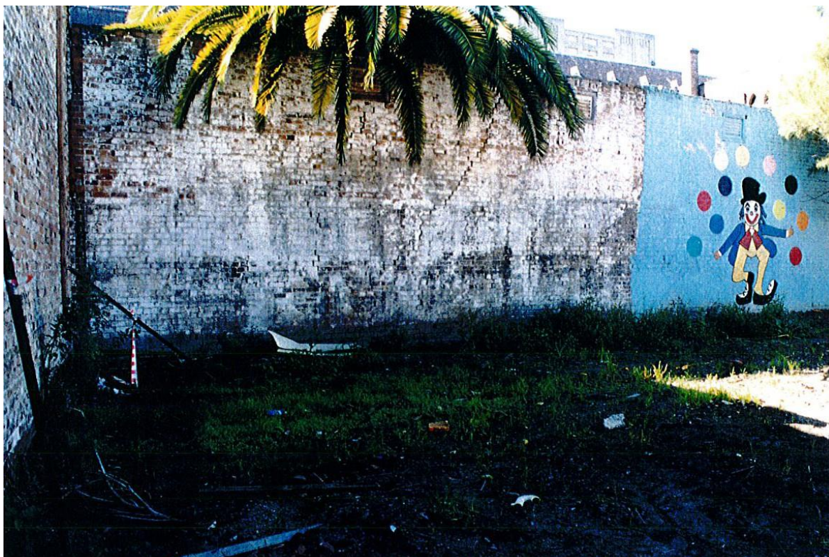
Figure 4.20: Eastern boundary wall showing severe cracking near palm tree. Photo taken looking east, BLKF 3.29.
