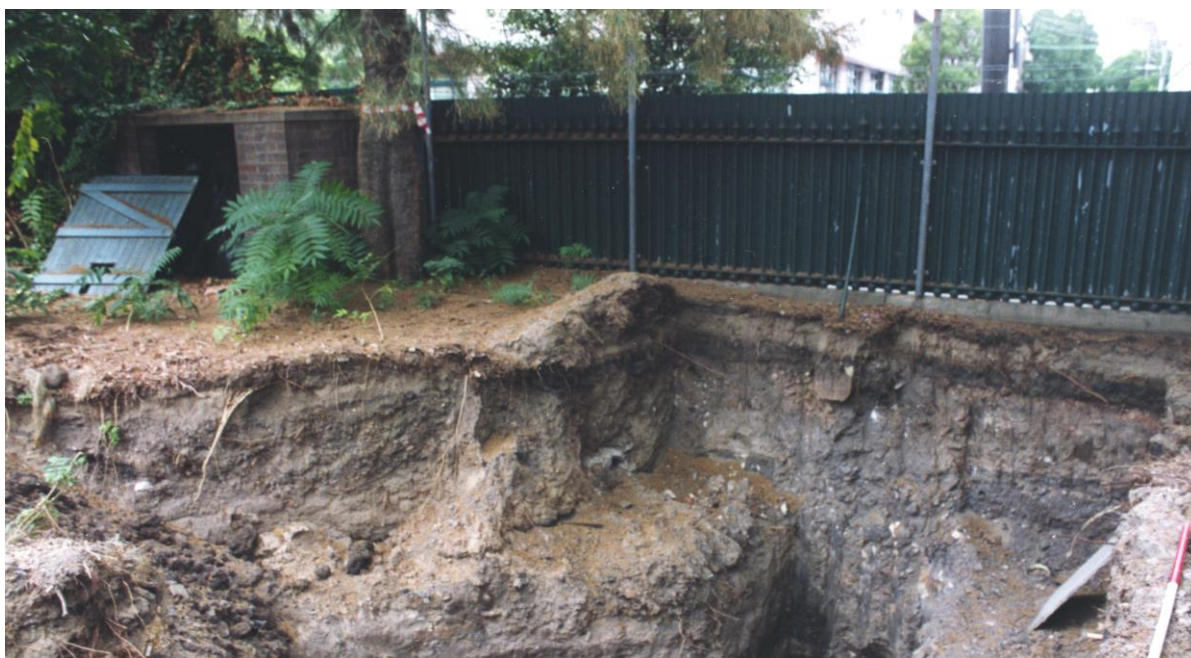
Figure 4.14: Southwest corner of gas main trench, Trench 1, in northern playground area. Photo taken looking southwest, BLKF 2:6.
