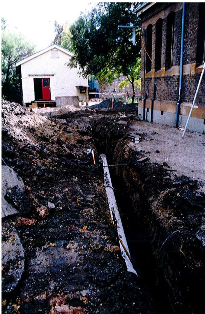
Figure 4.16: Trench 2 running down the centre of the site to the west of the Boys school. Photo taken looking north, BLKF 2.13, scale 1m.
