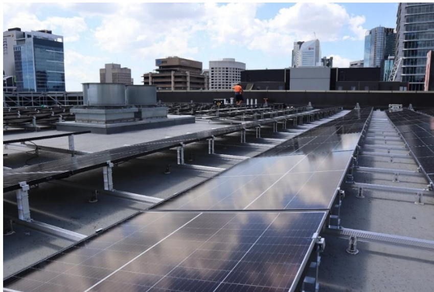
Figure 6 PV Solar on Roof
