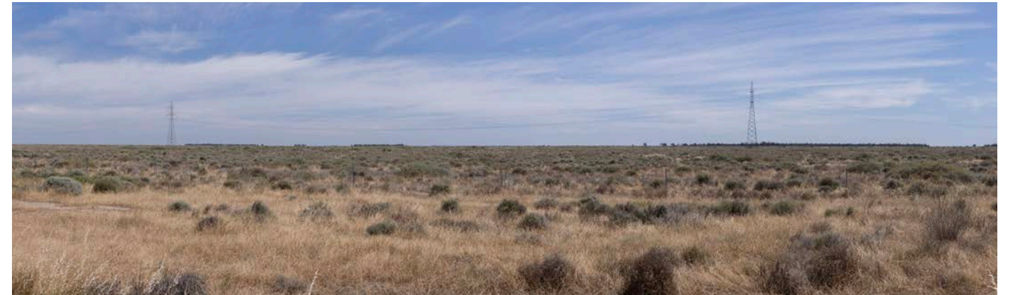
Image 06 Existing 220kV transmission line
