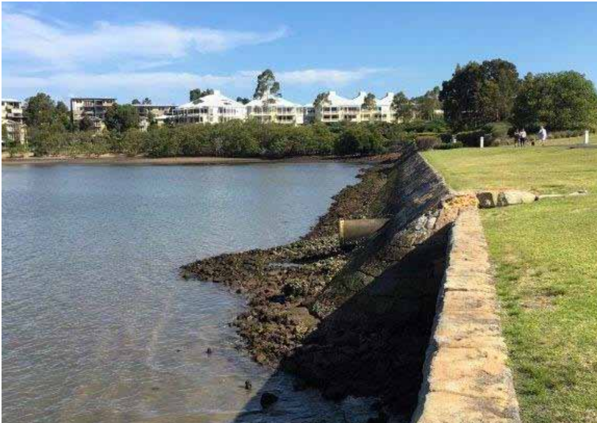
Figure 8.2. Sloped seawall and rubble along SW side of Kendall Bay
