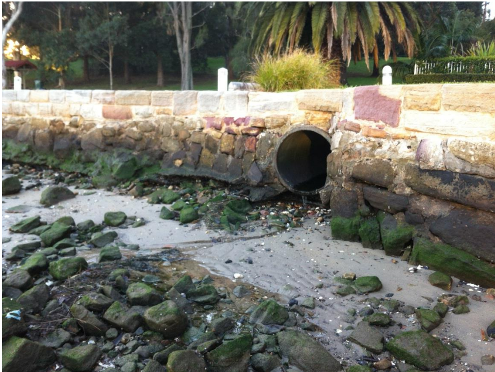
Figure 22: Stormwater outlet discharging onto beach area in July 2016
