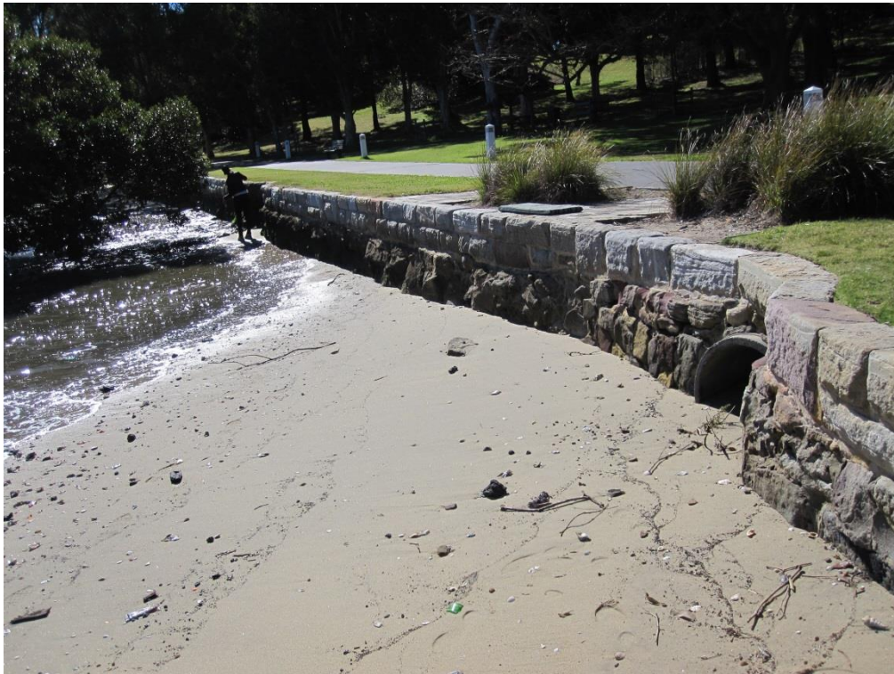
Figure 20: Sand covering underlying rock and partly blocking stormwater outlet in August 2012
