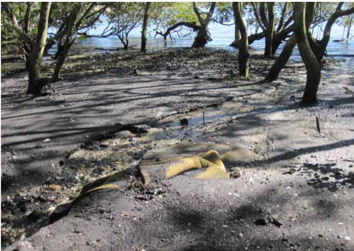
Figure 4.13. Shallow channel leading from 1650 mm stormwater outlet
