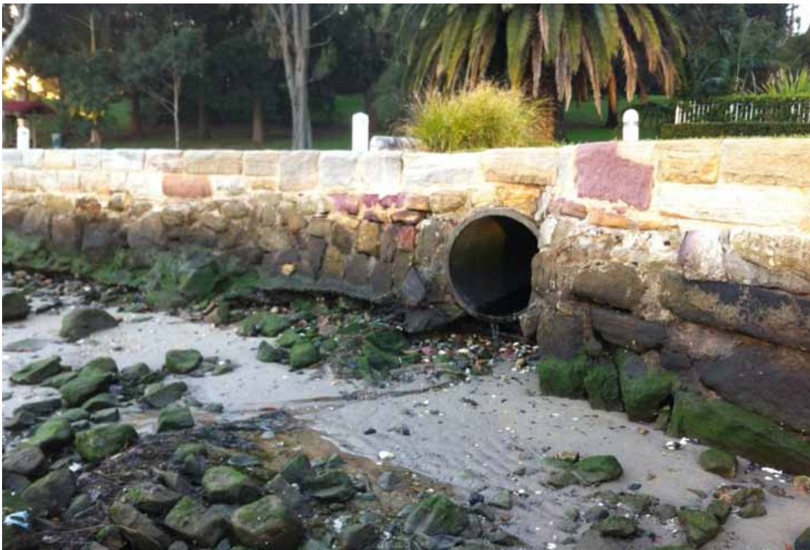
Figure 8.8. Stormwater outlet discharging onto beach in July 2016
