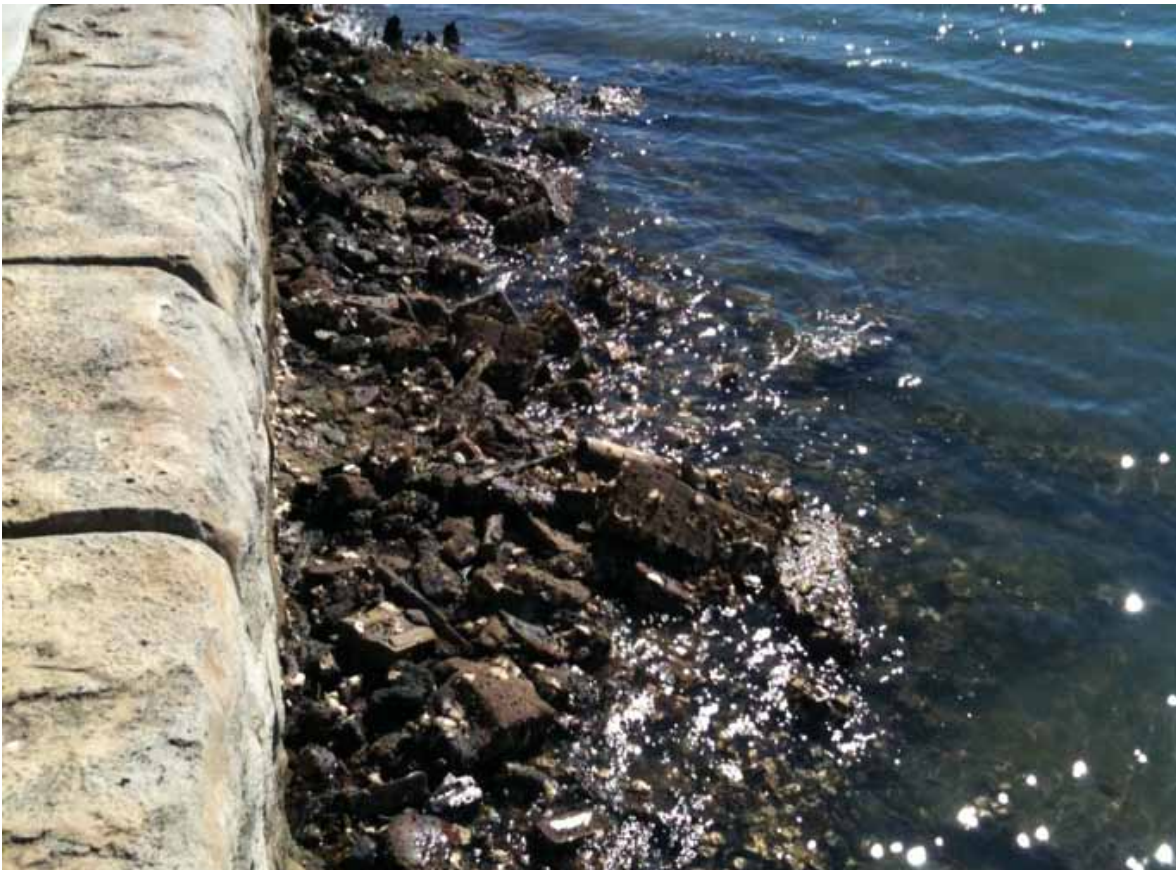
Figure 4.6. Rip-rap and rubble at location of demolished former coal wharf located within the proposed Remediation Area NA2+NA3.
