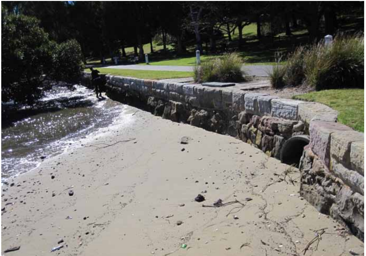
Figure 8.6. Sand covering underlying rock and partly blocking stormwater outlet in August 2012
