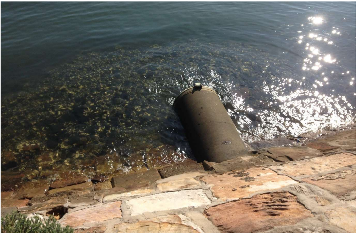
Plate 12-5: Stormwater drains and plume of oyster growth. (Source ERM 2014)
