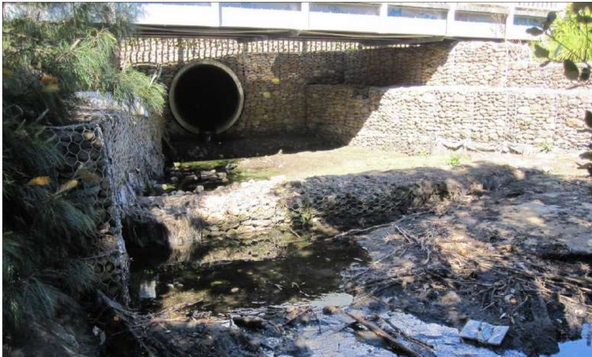
Plate 10-9: 1650 mm stormwater outlet at the head of Kendall Bay (Source: JBS&G 2017)
