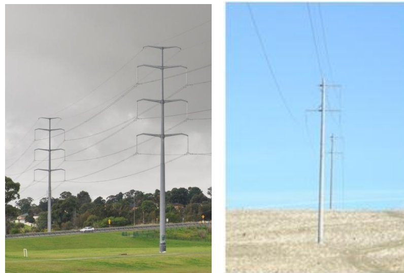
330kV double circuit steel poles
