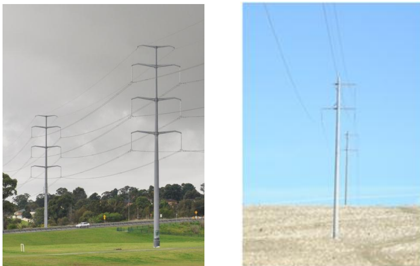
Figure 4-6 Typical overhead transmission line configurations: 330kV double circuit steel poles (left) 132kV single circuit concrete (right)
