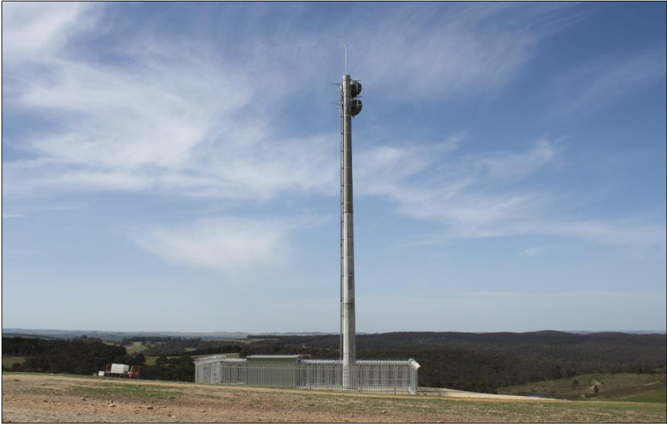
Example microwave communication tower
