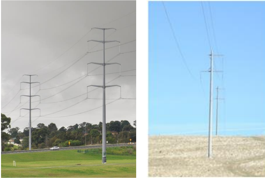
Figure 7-1 Typical overhead transmission line configurations - 330kV double circuit steel poles (left) 132kV single circuit concrete poles (right)
