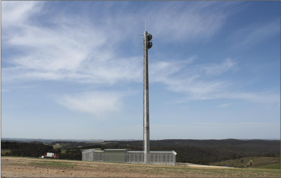
Example microwave communication tower
