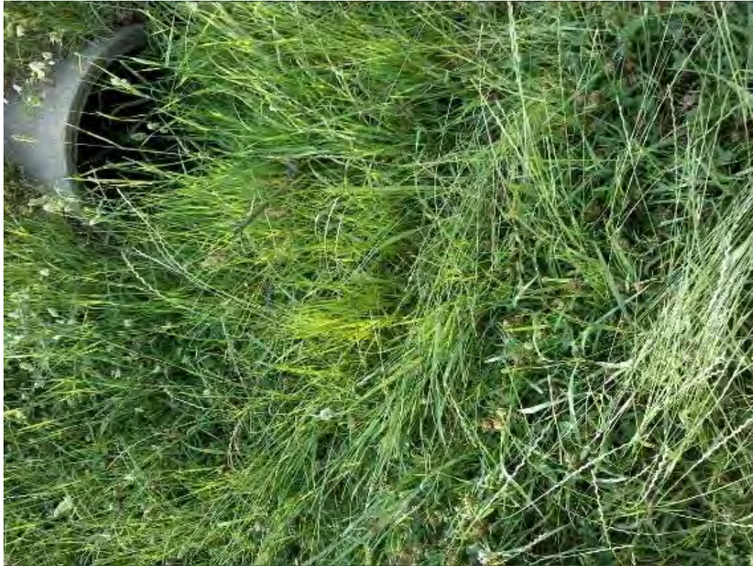
S059 – 600mm Pipe Culvert no headwall
