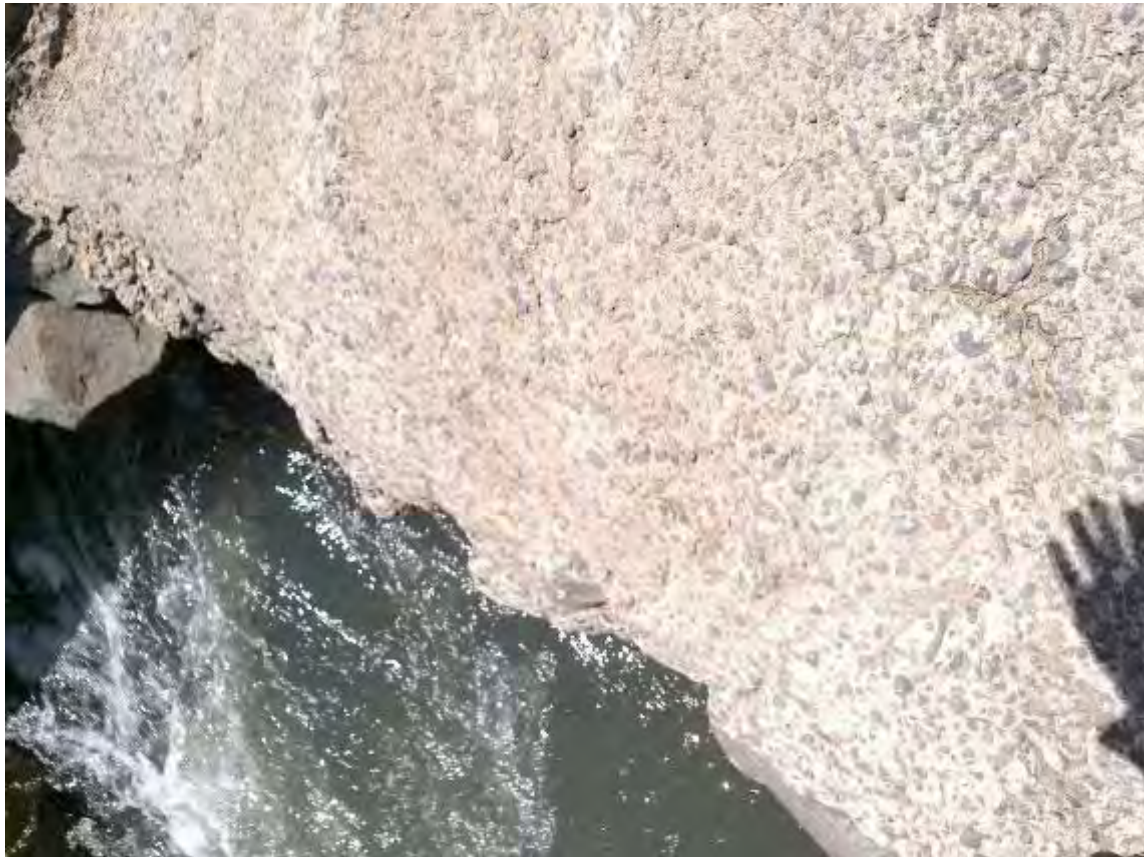
S025 – Edge of culvert is worn.
