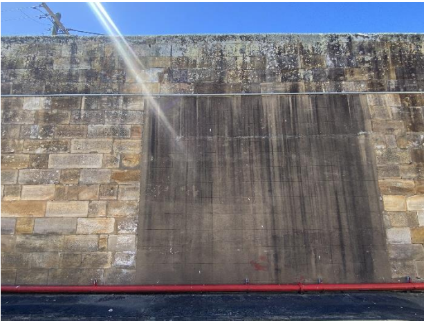
Figure 17 – Northern wall, interior showing render patch.
