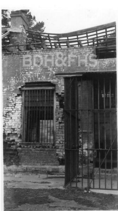
Figure A- 319 - Damaged section of Berrima Gaol, undated.
