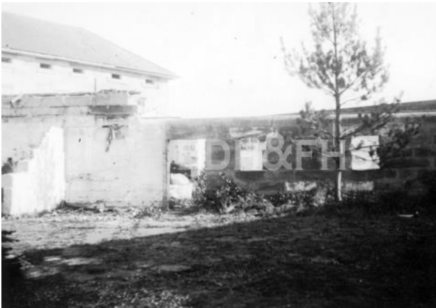
Figure A- 251 - Berrima Gaol, 1944. Photo shows one of the cell blocks in a state of disrepair and the yard very overgrown prior to work to establish Berrima Training Centre.
