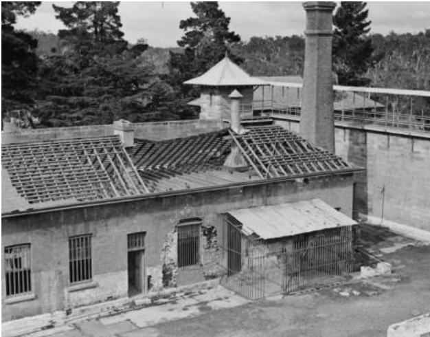
Figure 186 – Photograph of Dilapidated c.1839 outbuildings along the original entrance wall of Berrima Gaol, looking towards the former kitchen and bakehouse with chimney, observation tower and catwalk, 15 May 1932.
