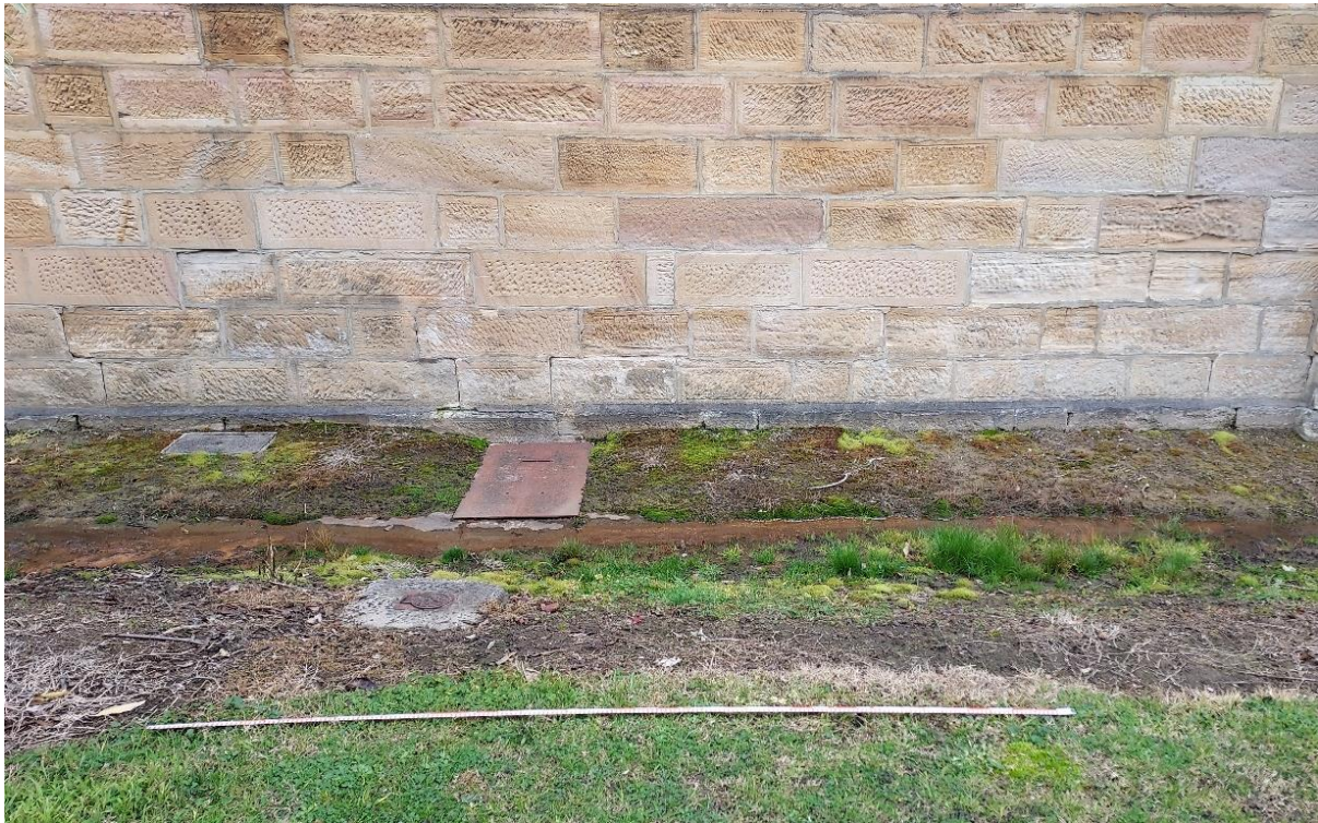
Figure 7.16 South-facing view of underground amenities along drainage channel (2 m scale).
