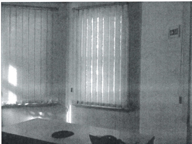
Photo No: J145125-BCC001-Photo090 Result: Lead (Paint) - Previously Sampled Positive Building/Level: 038 Admin/Governor-Ground Level Room/Location: All rooms-Throughout Feature/Material: Window Frame-Lower Paint System/s
