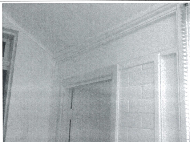
Photo No: J145125-BCC001-Photo102 Result: Asbestos - Previously Sampled Positive Building/Level: 038 Admin/Governor-Ground Level Room/Location: South-west Corridor-South Wall Feature/Material: Wall Covering-Fibre Cement Sheetting
