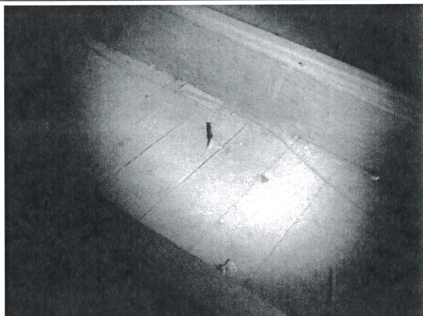
Photo No: J145125-BCC001-Photo098 Result: Lead (Dust) - Previously Sampled Positive Building/Level: 038 Admin/Governor-Ground Level Room/Location: Ceiling Space-Throughout Feature/Material: On Top of Ceiling-Dust - Lead
