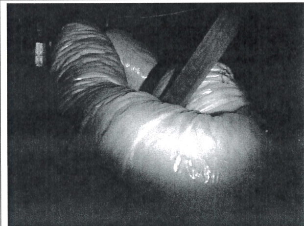
Photo No: J145125-BCC001-Photo096 Result: SMF - Positive Building/Level: 038 Admin/Governor-Ground Level Room/Location: Ceiling Space-Throughout Feature/Material: Ductwork Insulation-Insulation Material
