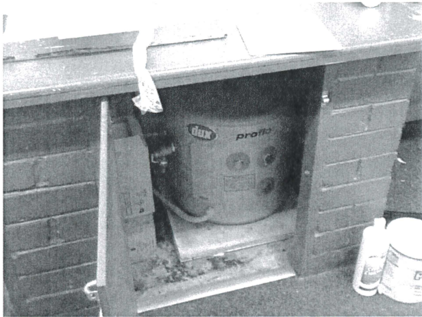
Photo No: J145125-BCC001-Photo051 Result: SMF - Presumed Positive Building/Level: 033 Maintenance/Teach/Welfare/P&P etc-Ground Level Room/Location: Maintenance-Office Feature/Material: Hot Water Heater-Insulation Material
