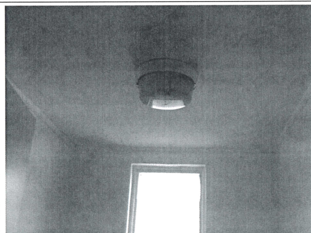
Photo No: J145125-BCC001-Photo103 Result: Asbestos - Previously Sampled Positive Building/Level: 038 Admin/Governor-Ground Level Room/Location: Toilet-South Feature/Material: Ceiling-Fibre Cement Sheetting
