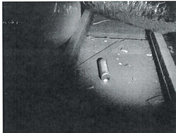
Photo No: J145125-BCC001-Photo097 Result: Lead (Dust) - Previously Sampled Positive Building/Level: 038 Admin/Governor-Ground Level Room/Location: Ceiling Space-Throughout Feature/Material: On Top of Ceiling-Dust - Lead
