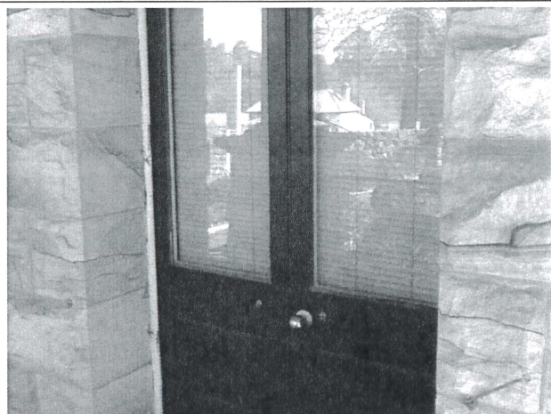
Photo No: J145125-BCC001-Photo070 Result: Lead (Paint) - Previously Sampled Positive Building/Level: 018 Oberon House-Ground Level Room/Location: Throughout-Doors Feature/Material: Door & Frame-Lower Paint System/s
