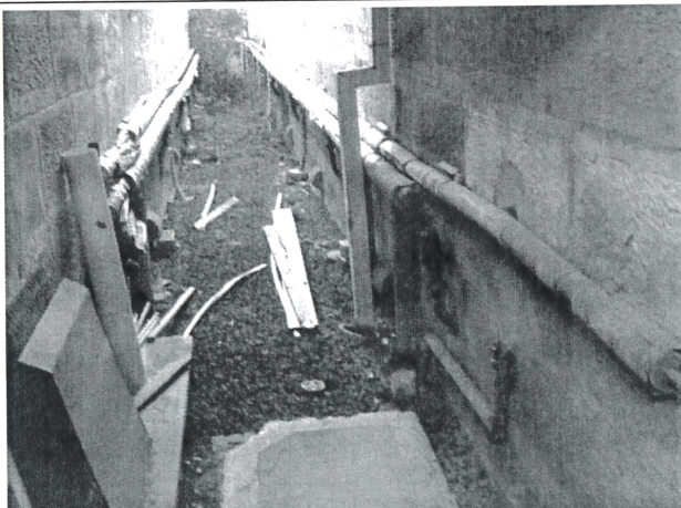
Photo No: J145125-BCC001-Photo050 Result: SMF - Positive Building/Level: 033 Maintenance/Teach/Welfare/P&P etc-Ground Level Room/Location: Maintenance-Northern Service Corridor Feature/Material: Pipework Insulation-Insulation Material
