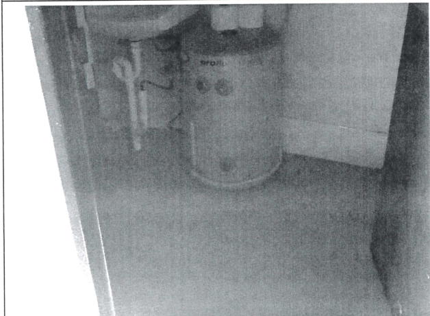
Photo No: J145125-BCC001-Photo038 Result: SMF - Presumed Positive Building/Level: 016 Industries Building-Ground Level Room/Location: Officers Toilet-Throughout Feature/Material: Hot Water Heater-Insulation Material
