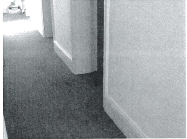
Photo No: J145125-BCC001-Photo088 Result: Lead (Paint) - Previously Sampled Positive Building/Level: 038 Admin/Governor-Ground Level Room/Location: All rooms-Throughout Feature/Material: Timber Work-Lower Paint System/s
