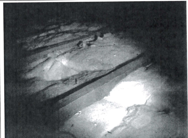
Photo No: J145125-BCC001-Photo052 Result: SMF - Positive Building/Level: 033 Maintenance/Teach/Welfare/P&P etc-Ground Level Room/Location: Maintenance-Ceiling Space Feature/Material: Insulation-Insulation Batt/s
