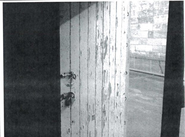
Photo No: J145125-BCC001-Photo057 Result: Lead (Paint) - Positive Building/Level: 032 Store-Ground Level Room/Location: Entry Door- Feature/Material: Door & Frame-Upper & Lower Paint System/s
