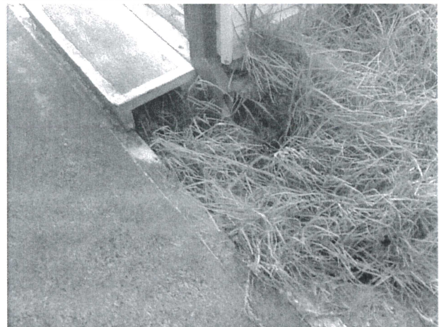
Photo No: J145125-BCC001-Photo065 Result: Asbestos - Previously Sampled Positive Building/Level: 036 Recept/Roster/Segro-Ground Level Room/Location: In Ground-Drainage Pipe Feature/Material: Pipe-Moulded Fibre Cement
