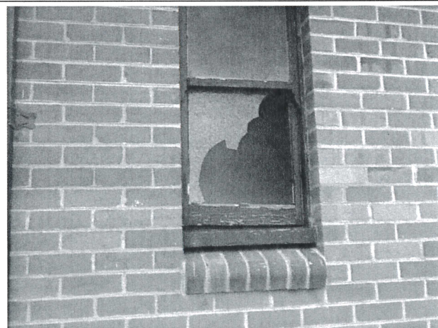
Photo No: J145125-BCC001-Photo075 Result: Lead (Paint) - Previously Sampled Positive Building/Level: 019 Dangerous Goods Store-Ground Level Room/Location: Exterior-Windows Feature/Material: Window Frame-Lower Paint System/s
