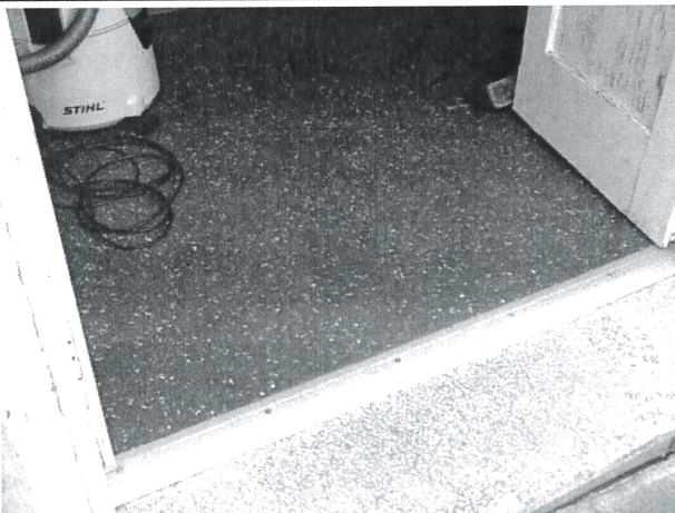
Photo No: J145125-BCC001-Photo022 Result: Asbestos - Previously Sampled Positive Building/Level: 003 MDI/DEP GOV/BOX VISITS-Ground Level Room/Location: Entrance to Staff Room-Floor under carpet & linoleum Feature/Material: Floor-Fibre Cement Sheetting
