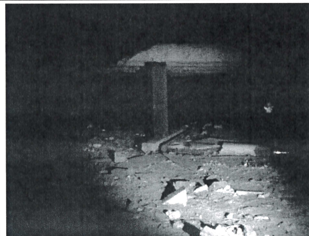
Photo No: J145125-BCC001-Photo076 Result: Lead (Dust) - Previously Sampled Positive Building/Level: 019 Dangerous Goods Store-Ground Level Room/Location: Ceiling Space-Throughout Feature/Material: On Top of Ceiling-Dust - Lead
