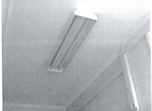
Photo No: J145125-BCC001-Photo018 Result: PCB - Presumed Positive Building/Level: 003 MDI/DEP GOV/BOX VISITS-Ground Level Room/Location: Main Switchroom-Throughout Feature/Material: Fluorescent Light Fitting - Double Tube-Capacitor
