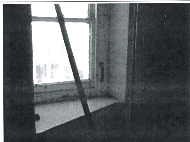
Photo No: J145125-BCC001-Photo003 Result: Lead (Paint) - Previously Sampled Positive Building/Level: 001 Gatehouse -All Levels Room/Location: All rooms-Throughout Feature/Material: Window Frame-Upper & Lower Paint System/s
