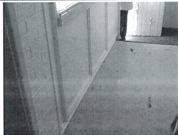
Photo No: J145125-BCC001-Photo101 Result: Asbestos - Previously Sampled Positive Building/Level: 038 Admin/Governor-Ground Level Room/Location: South-west Corridor-Under Windows Feature/Material: Infill Panels - Low Level-Fibre Cement Sheetting
