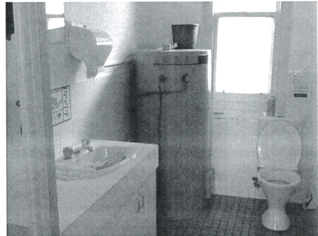
Photo No: J145125-BCC001-Photo093 Result: SMF - Presumed Positive Building/Level: 038 Admin/Governor-Ground Level Room/Location: Bathroom-North Feature/Material: Hot Water Heater-Insulation Material
