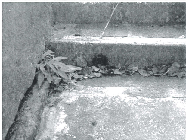
Photo No: J145125-BCC001-Photo068 Result: Asbestos - Previously Sampled Positive Building/Level: 800 Outer Grounds-Ground Level Room/Location: Adjacent Main Entry-Buired under both sides of steps Feature/Material: Pipe-Moulded Fibre Cement
