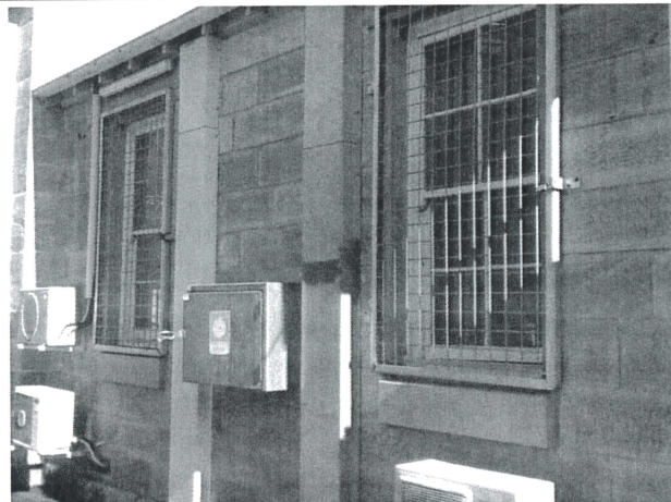
Photo No: J145125-BCC001-Photo025 Result: Lead (Paint) - Previously Sampled Positive Building/Level: 007 Area Case Manager-Ground Level Room/Location: Exterior-Surrounding Feature/Material: Window Frame-Upper & Lower Paint System/s
