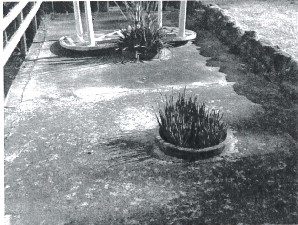
Photo No: J145125-BCC001-Photo085 Result: Asbestos - Previously Sampled Positive Building/Level: 017 Officers Amenities Building-Ground Level Room/Location: House-North Garden Feature/Material: Pit-Moulded Fibre Cement
