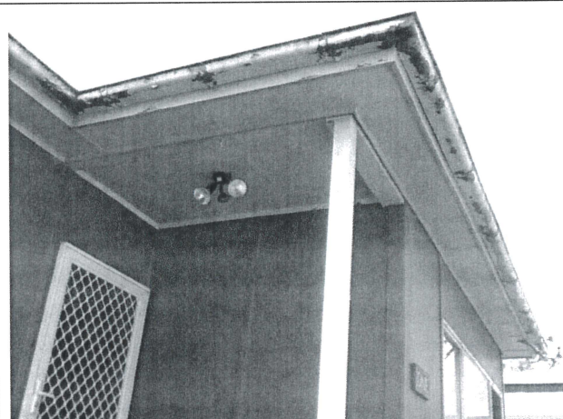
Photo No: J145125-BCC001-Photo083 Result: Asbestos - Previously Sampled Positive Building/Level: 017 Officers Amenities Building-Ground Level Room/Location: House-Surrounding Feature/Material: Eaves-Fibre Cement Sheetting
