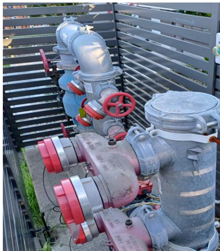
Image 18 and 19 improved signed and enclosed installations - Harris
