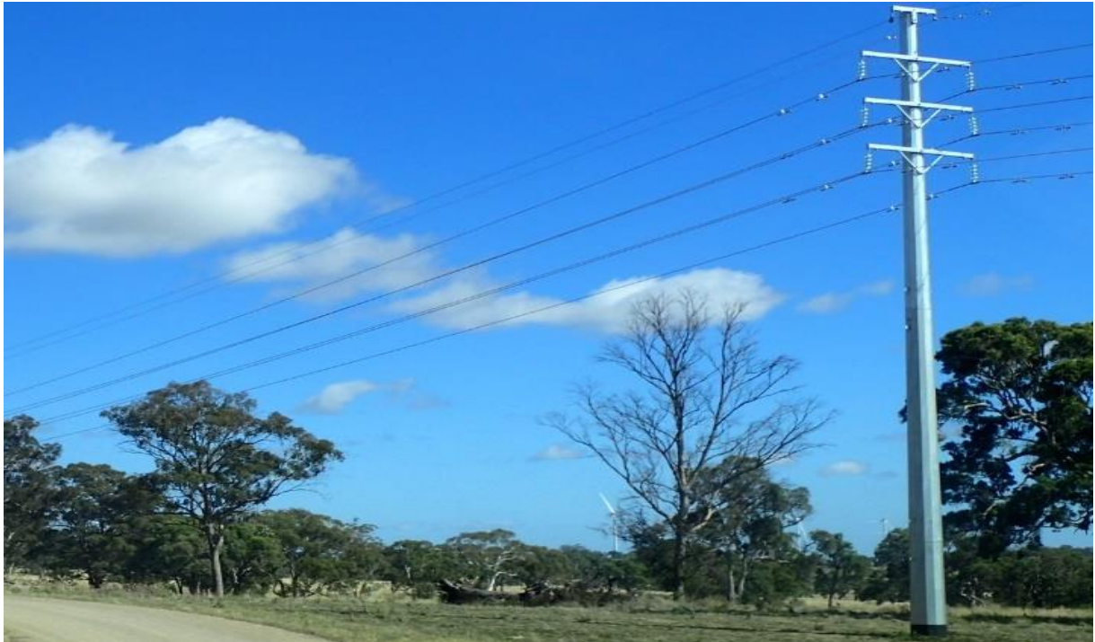
Figure 4-15: Double-circuit overhead 33 kV transmission line
