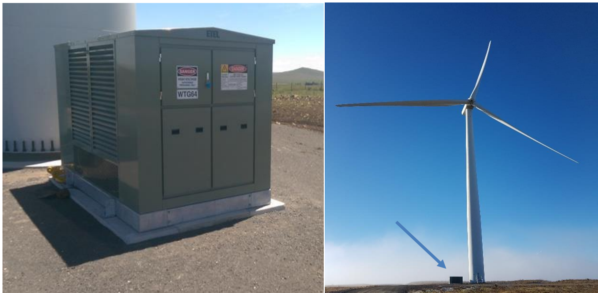
Figure 4-11: Example of a generator transformer located outside of the tower at Boco Rock wind farm
