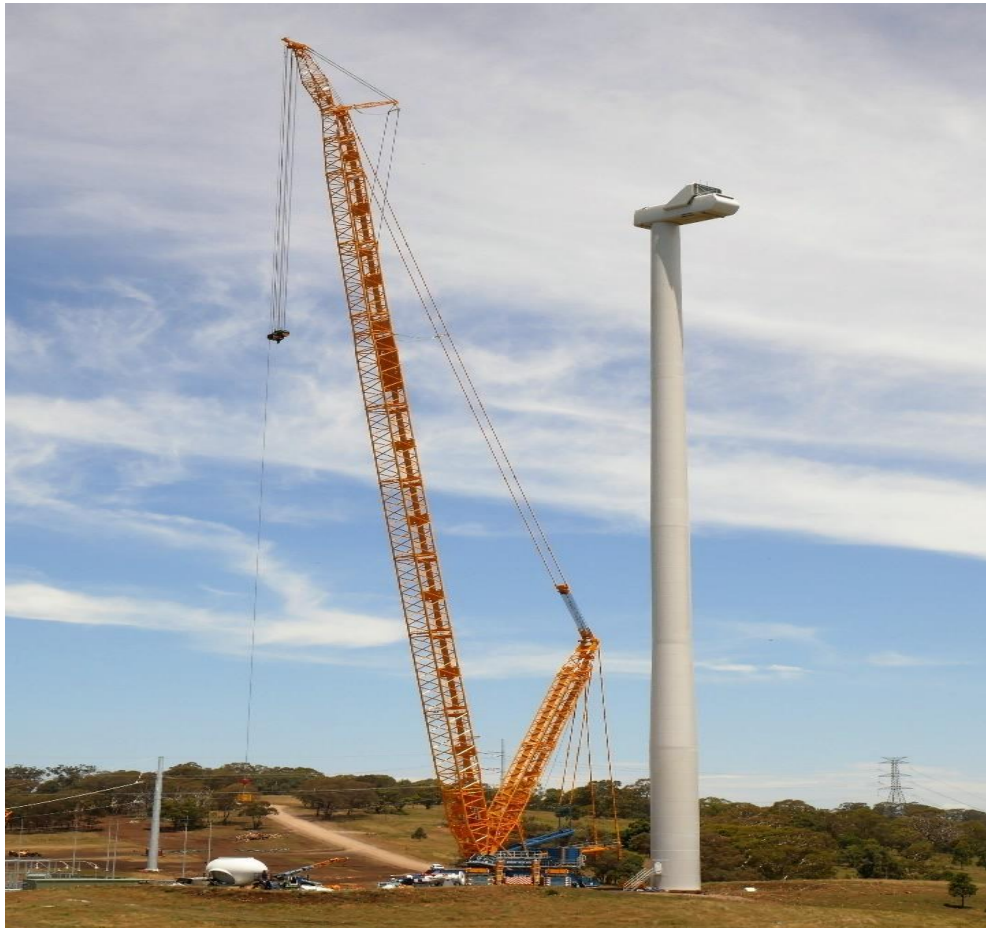
Figure 4-8: Example of a WTG tower with the nacelle mounted at Sapphire Wind Farm
