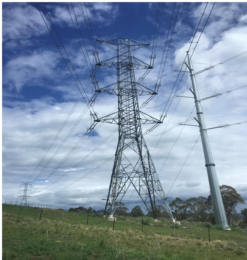
Figure 4-16: Example of double-circuit overhead 330 kV transmission line adjacent to a new single-pole substation tie-in
