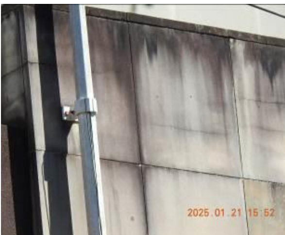
Figure 175 - Crack propagation through external wall
