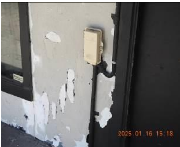
Figure 45 - Loss of material through external wall
