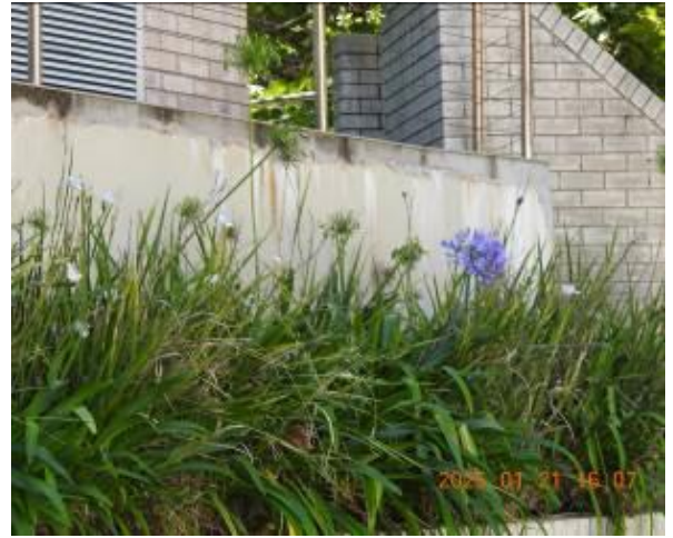
Figure 304 - Crack propagation through external wall
