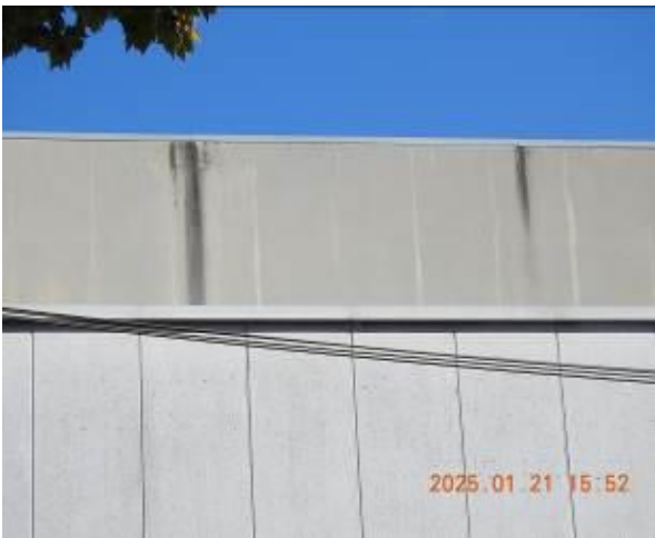
Figure 179 - Crack propagation through external wall
