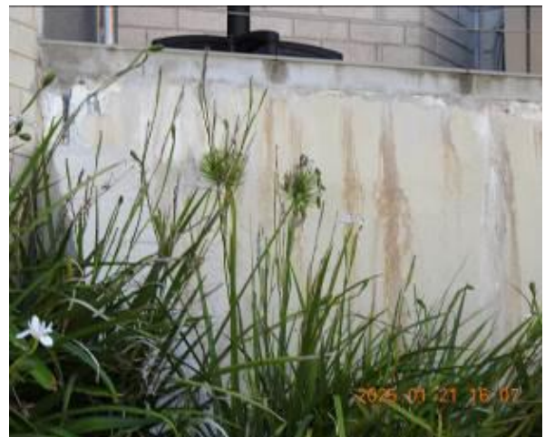
Figure 302 - Crack propagation through external wall
