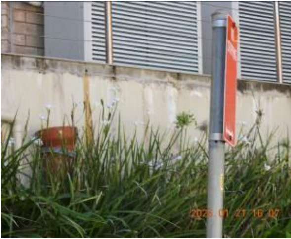
Figure 303 - Crack propagation through external wall
