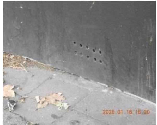
Figure 60 - Loss of material through external wall
