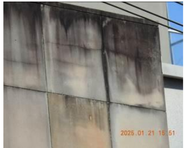
Figure 174 - Crack propagation through external wall
