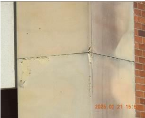
Figure 187 - Loss of material through external wall
