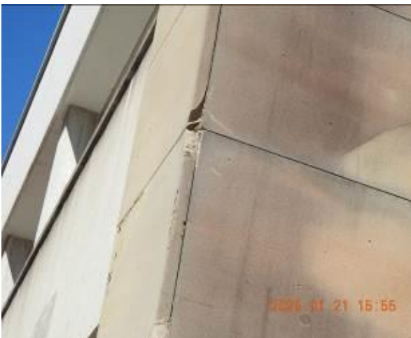
Figure 205 - Crack propagation and loss of material through external wall
