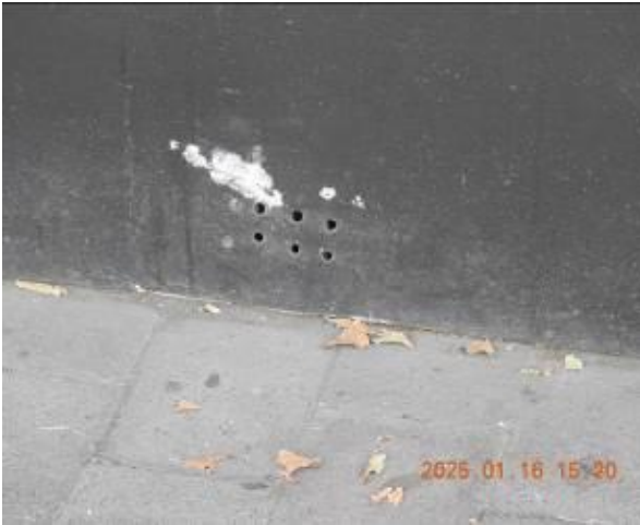
Figure 59 – Loss of material through external wall
