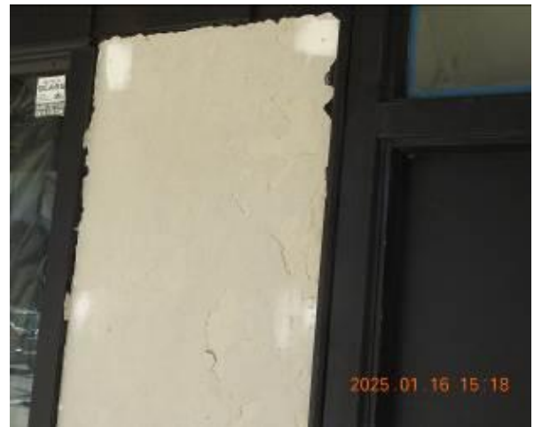
Figure 44 - Crack propagation through external wall
