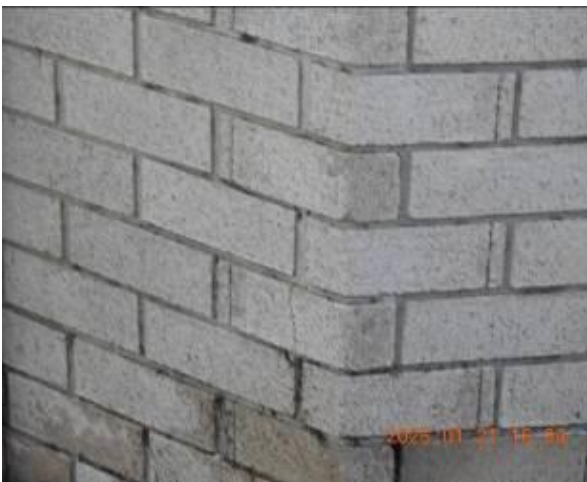
Figure 319 - Crack propagation through external wall
