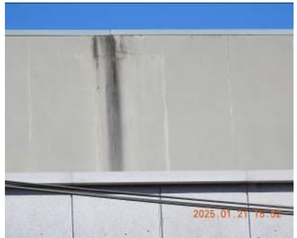
Figure 180 - Crack propagation through external wall
