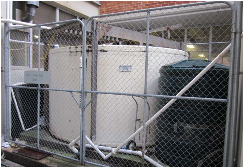
Photo 7 – Aboveground reservoir tank
