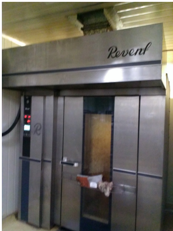
Figure A - 2: Electric oven
