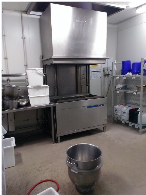
Figure A - 4: Dishwasher with overhead steam extraction system
