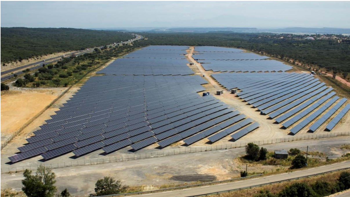
Figure 1-4 11MWp solar project constructed in Rochefort du Gard, France (Source Neoen Australia, 2014)
