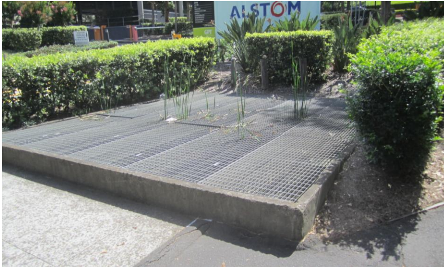
Figure 6: SWQCP downstream discharge point – junction pit at ‘Crossing 1’ culverts to Bennelong Pond ‘forebay’
