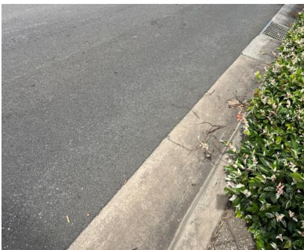
Figure 51 – General view of road pavement. Cracking to gutter.
