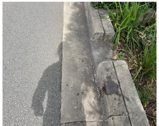
Figure 120 – Cracking to gutter.
