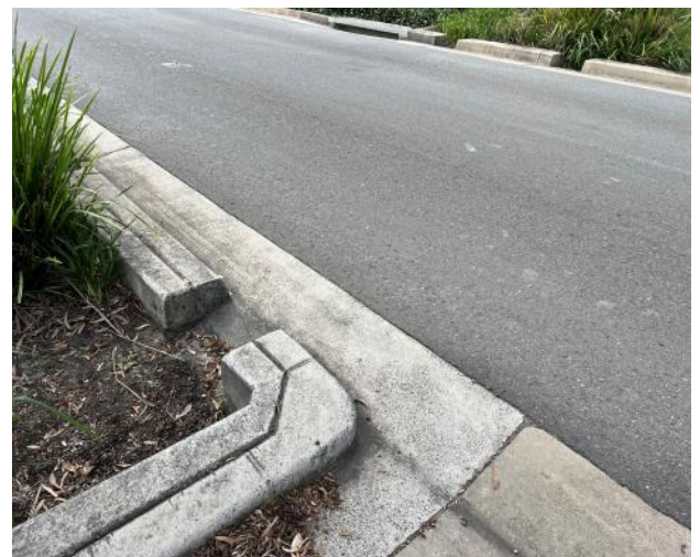
Figure 30 – Current condition of kerb and gutter.
