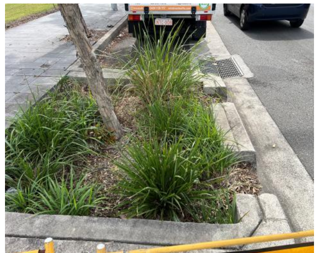
Figure 18 – Current condition of tree pit.
