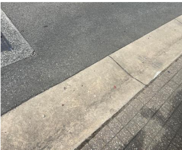
Figure 65 – Current condition of gutter.
