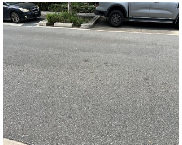
Figure 90 – Current condition of road pavement.
