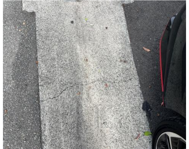
Figure 116 – Cracking to road gutter.
