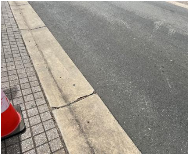
Figure 55 – General view of road pavement. Cracking to gutter.
