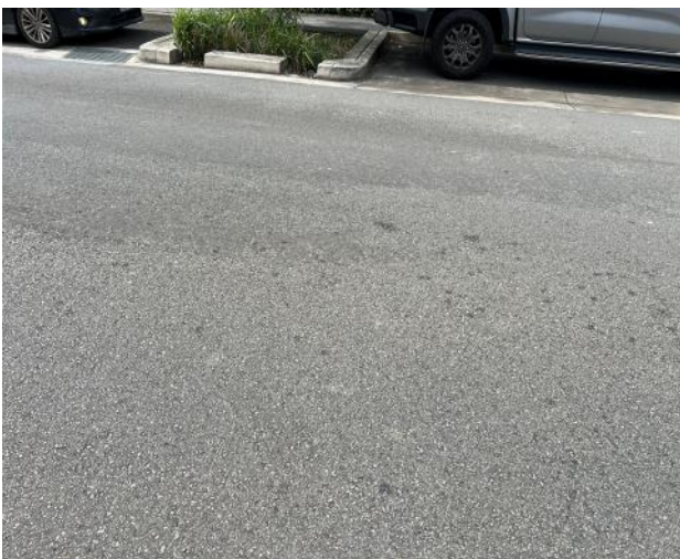
Figure 17 – Current condition of road pavement.
