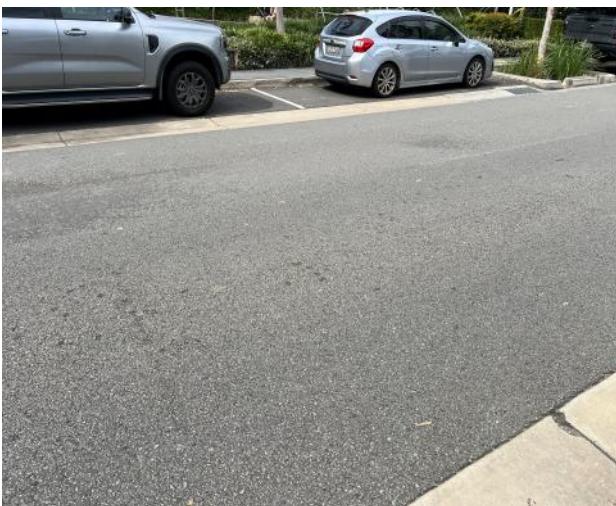
Figure 89 – Current condition of road pavement.
