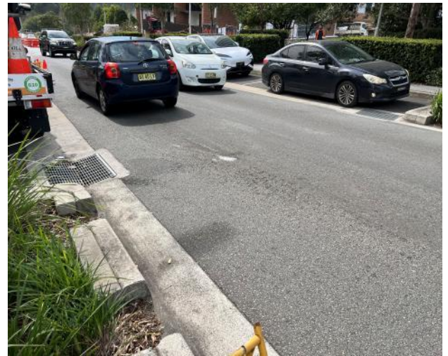
Figure 20 – Current condition of road pavement.
