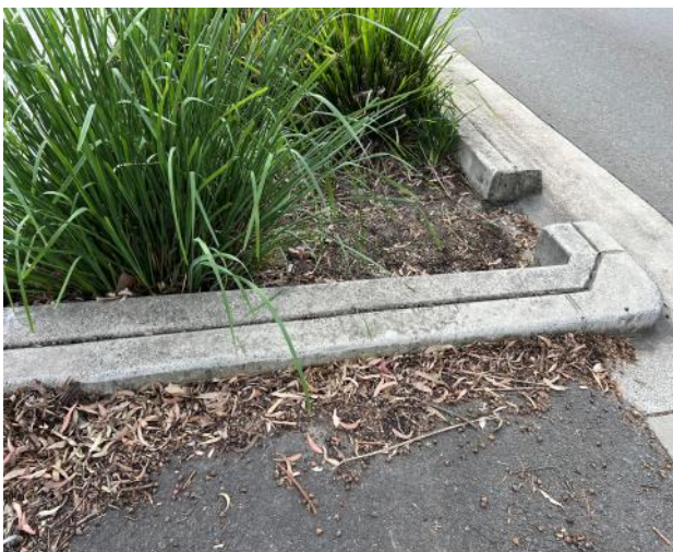
Figure 29 – Current condition of kerb around tree/shrub pit.
