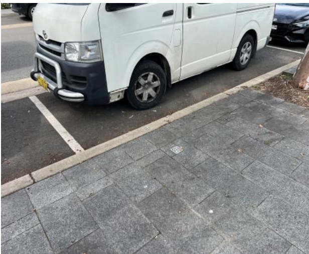
Figure 99 – Current condition of council footpath.
