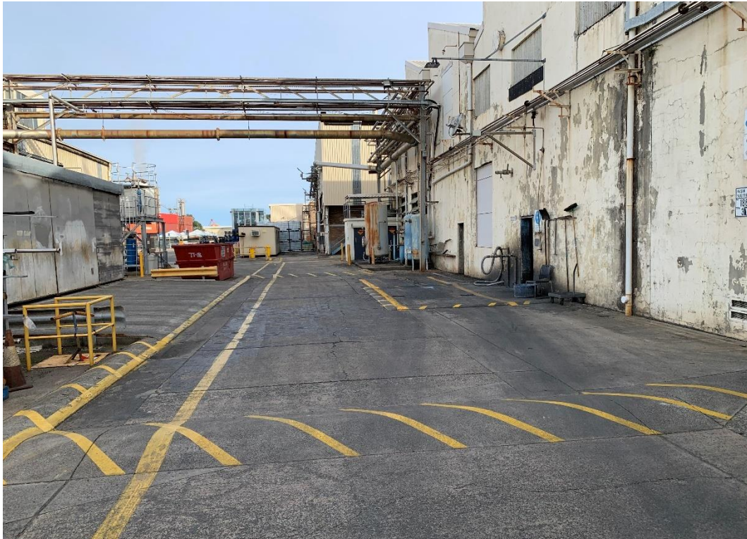
Photo 91: 29a Bunded Fill Point On East Side of Emulsions Plant Storage Building (Looking South)
