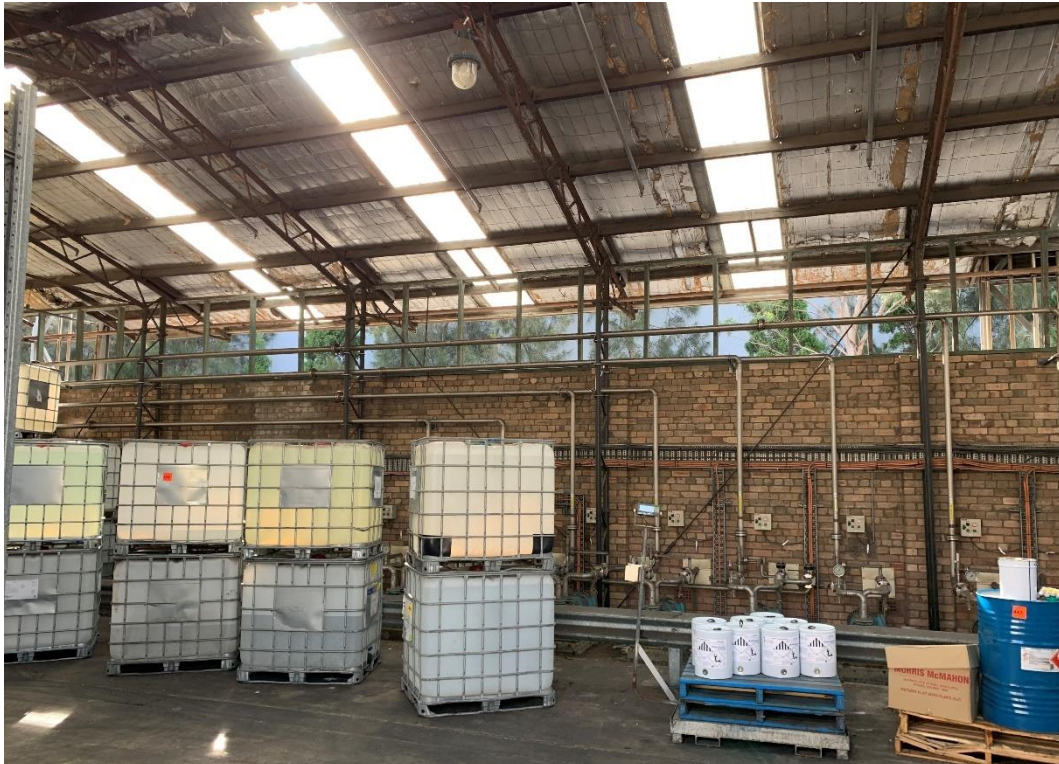
Photo 33: Northern UST Farm Pump Room
