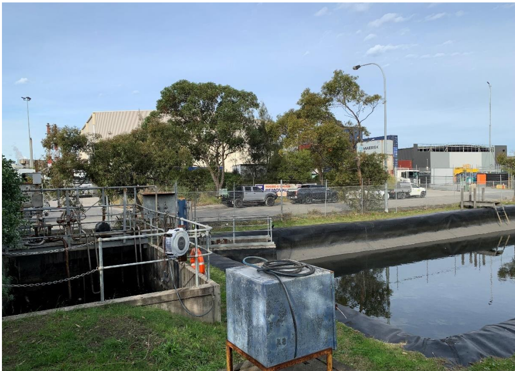
Photo 124: Stormwater Interception Pit, Disposal Point and Overflow Basin
