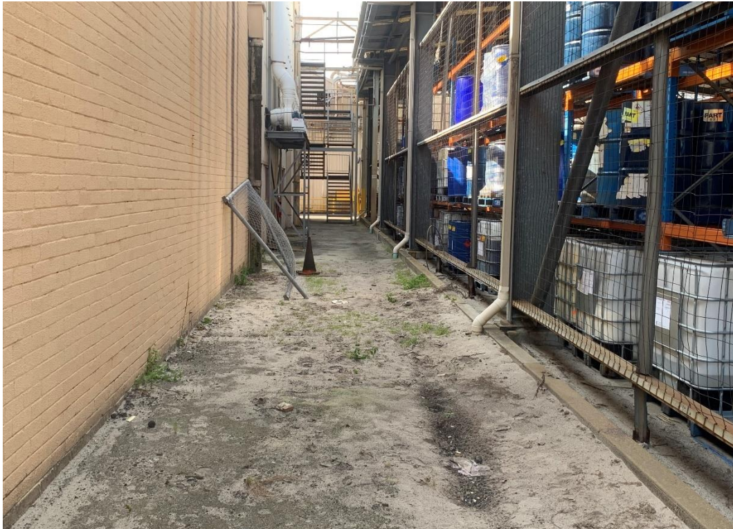
Photo 59: Unsealed Area Between Production Office and Drum Storage Building
