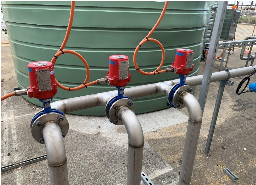
Photo 64: Groundwater Remediation System
