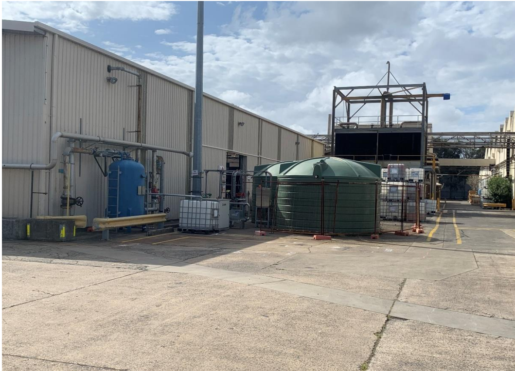
Photo 63: Groundwater Remediation System (Looking North)
