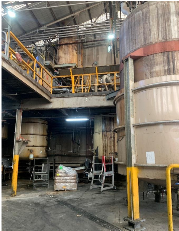
Photo 19: Alkyd Resin Plant Thinning Room
