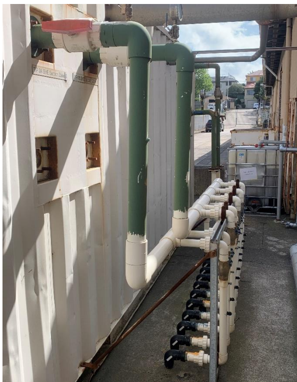
Photo 65: Boundary Remediation System - Soil Vapour Treatment System
