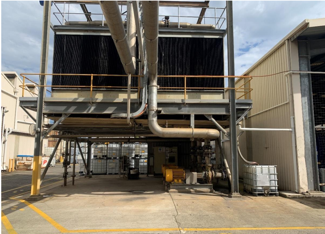
Photo 57: Cooling Tower In Central Area of Site
