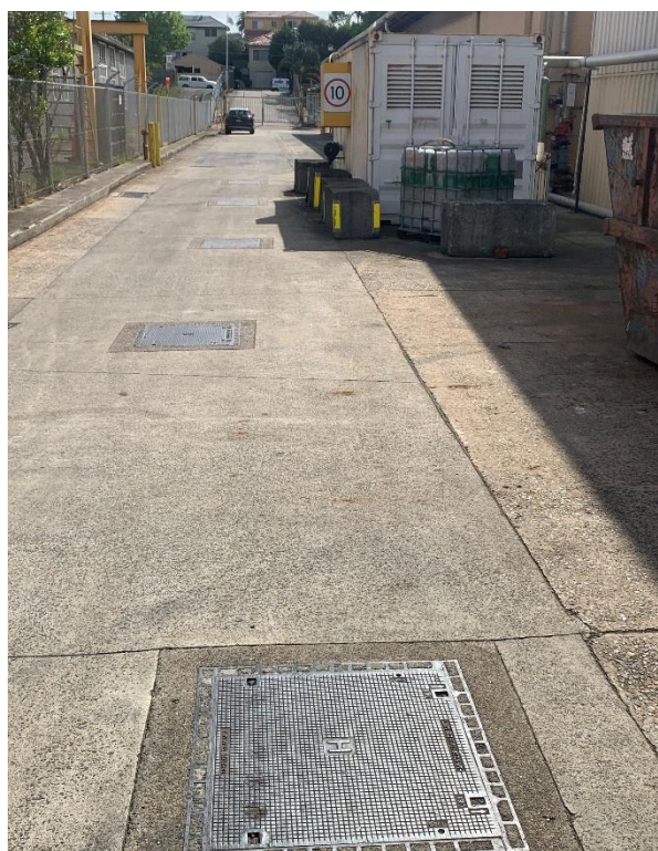
Photo 62: Boundary Remediation System - Wells and Soil Vapour Treatment System (Looking West)
