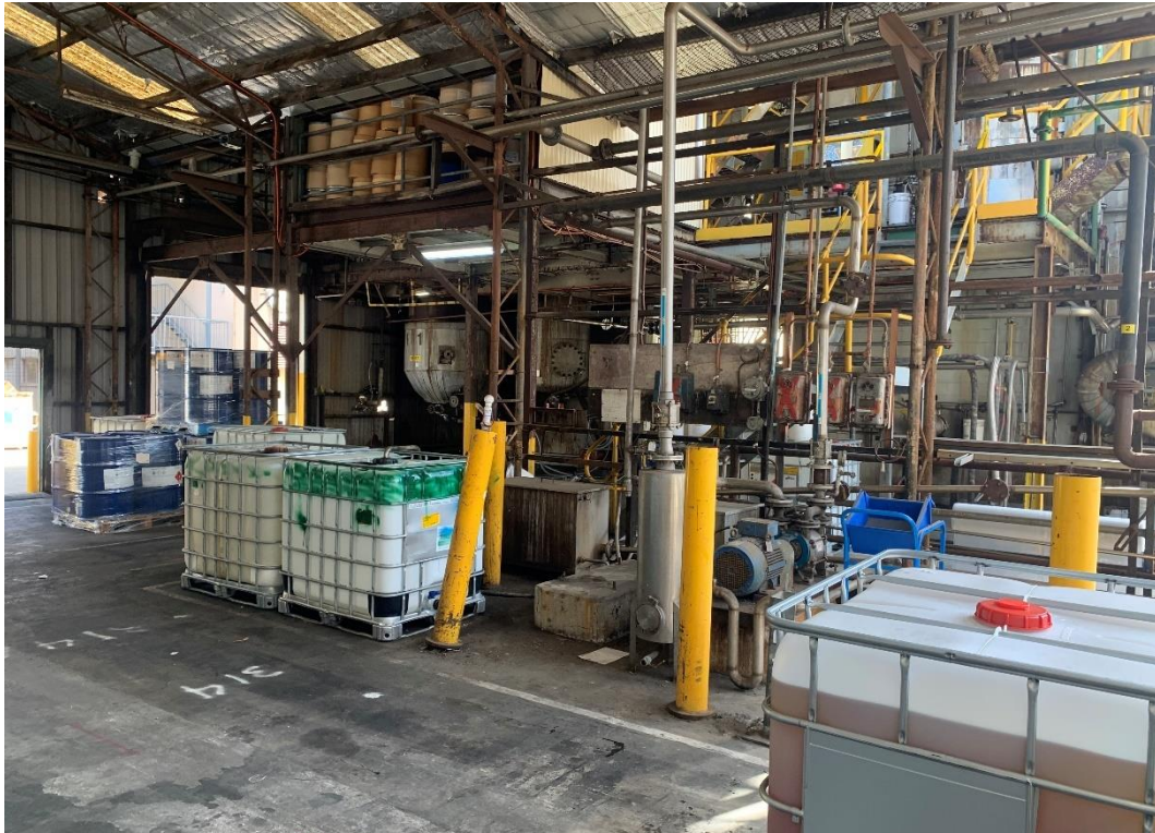
Photo 53: Beckamine Plant (East)
