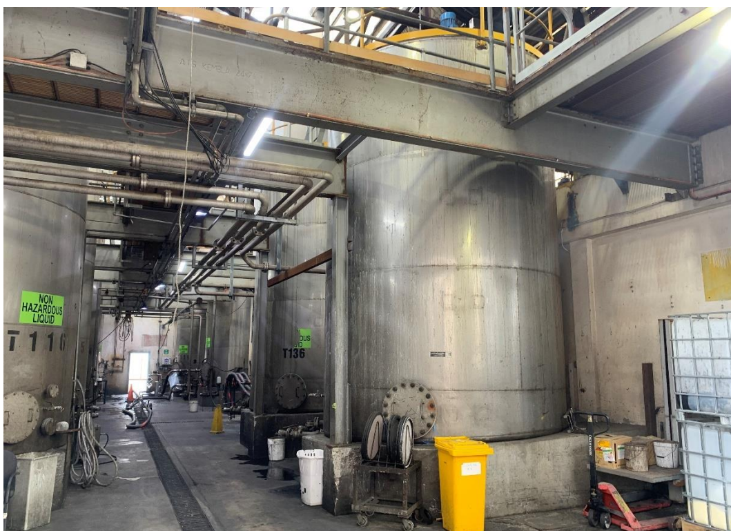
Photo 72: Emulsions Plant Storage Building ASTs (Looking East)
