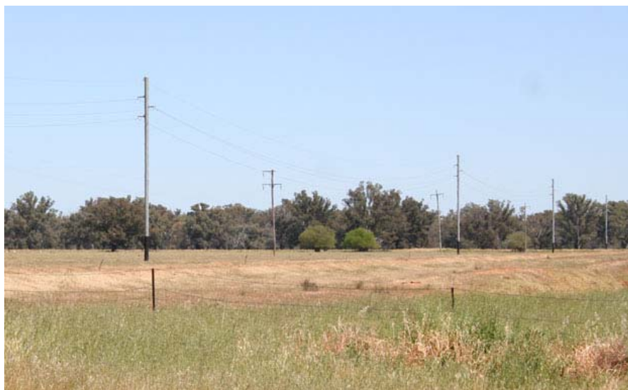
Figure 2-12 66kV transmission line recently installed by Essential Energy in the vicinity (in foreground)
