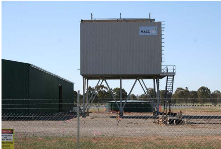
Figure 2-9 Air-cooled condenser at the Vast Solar 6MW pilot plant at Jemalong
