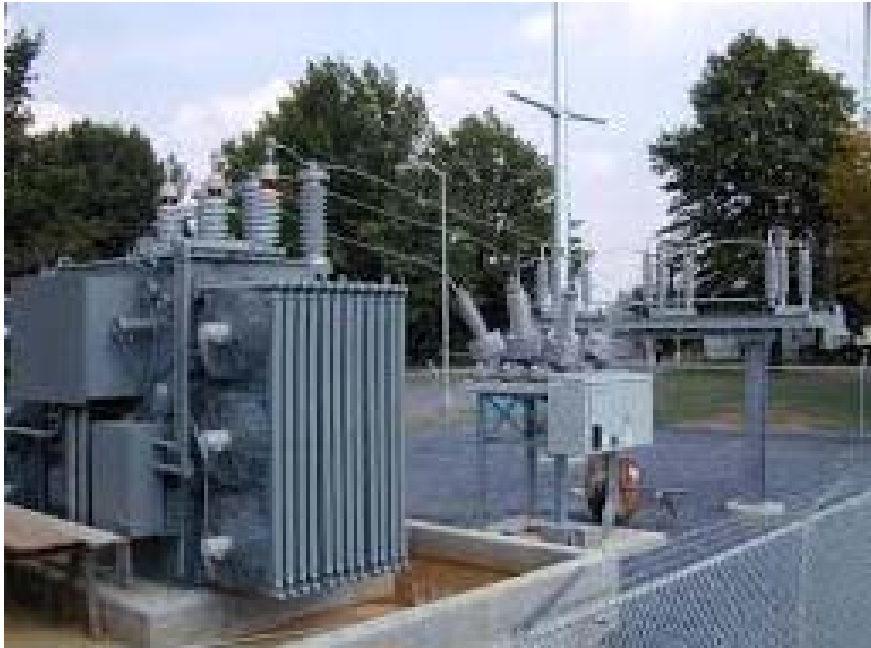
Figure 2-10 Typical fenced transformer station showing transformer and switchgear
