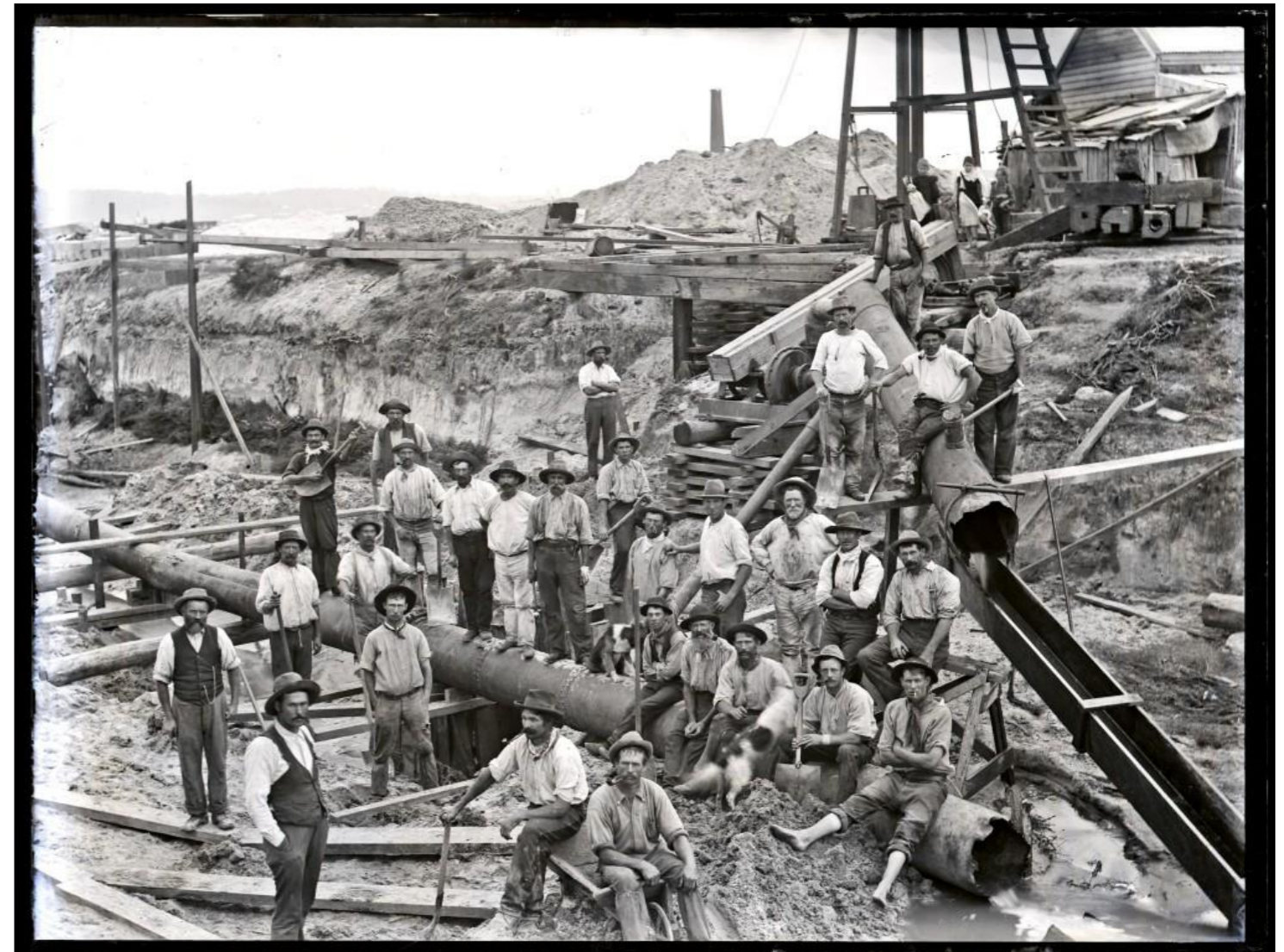
Figure 8: Image taken from Artefact Report - "Drain construction workers at Broadmeadow, NSW, 6 April 1900. University of Newcastle Cultural Collections."
