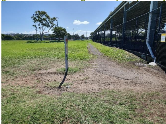
Figure 22. View west showing extent of exposed ground surface leading to an asphalt pathway.
