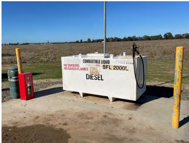
Photograph 7 - Onsite self-bunded 2000 L diesel above ground storage tank (AST).
