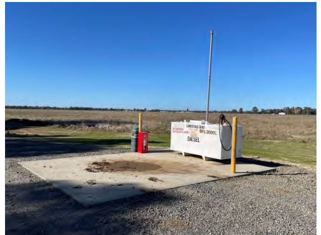
Photograph 8 - Onsite diesel AST with some staining on the concrete pad.
