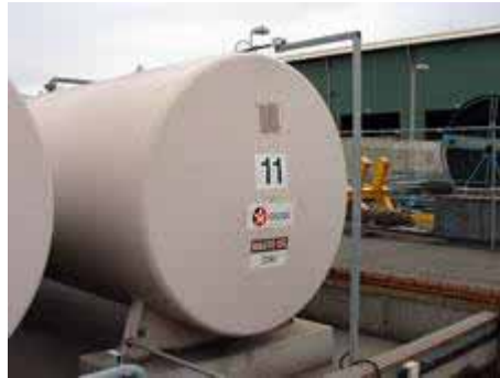
Bulk waste oil storage facility (fully bunded)
