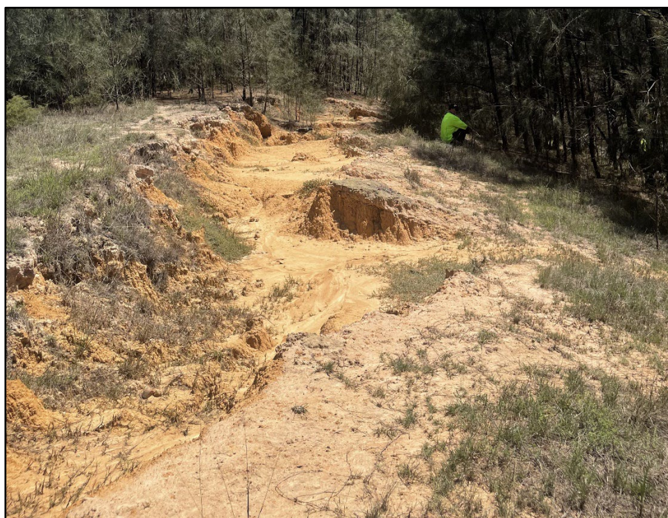
Erosion scour along Loder Creek
