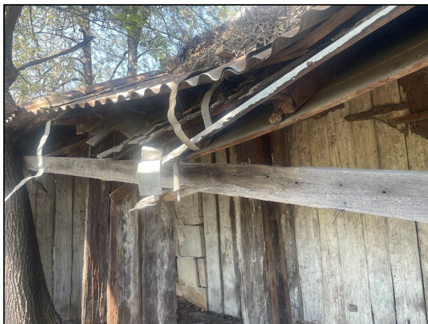
Increased slumping along eastern wall
