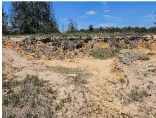
Figure 7: Erosion scar along the upper right-hand bank.
