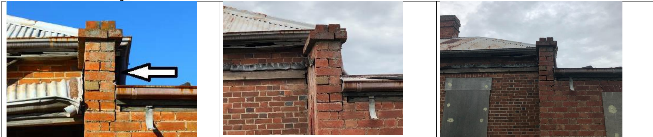
View of south-east of building (focus on top of wall) 2015-8: no discernible change 2018-20: no discernible change
