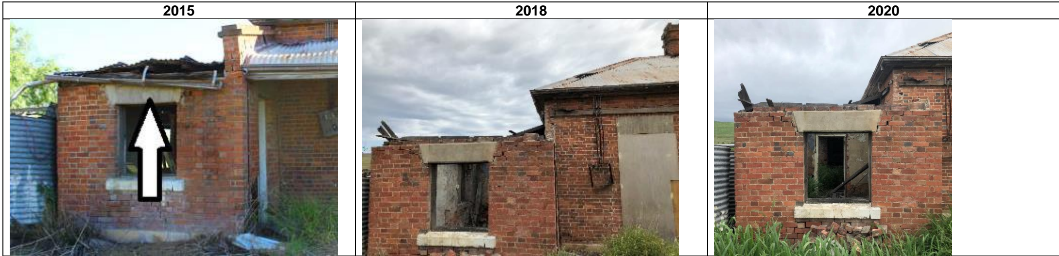
View of north-east of building (focus on skillion roof) 2015-8: roof framing, sheeting and guttering has collapsed 2018-20: no discernible change
