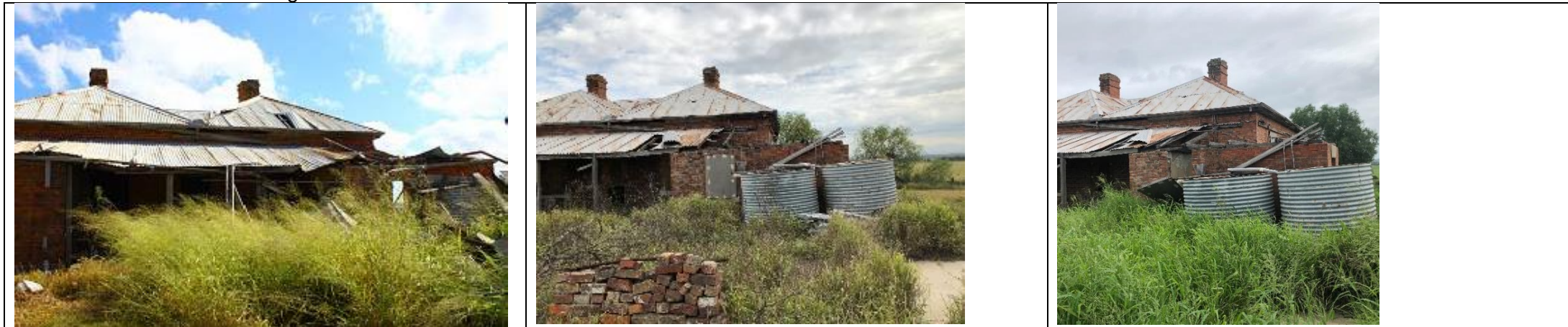
View of rear of building (focus on guttering) 2015-8: main roof holes repaired but northern section of skillion roof collapsed and guttering unchanged 2018-20: no discernible change, however vegetation regrowth evident
