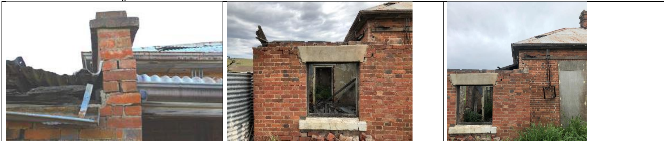
View of north-east of building (focus on top of wall) 2015-8: wall element has collapsed bricks stacked under window) 2018-20: no discernible change
