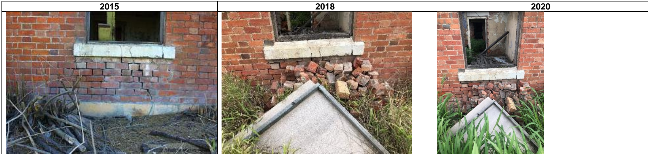
View of north-east corner of building (focus wall below window) 2015-8: bricks from roof above stacked in front of required repointing, window sheeting removed 2018-20: no discernible change
