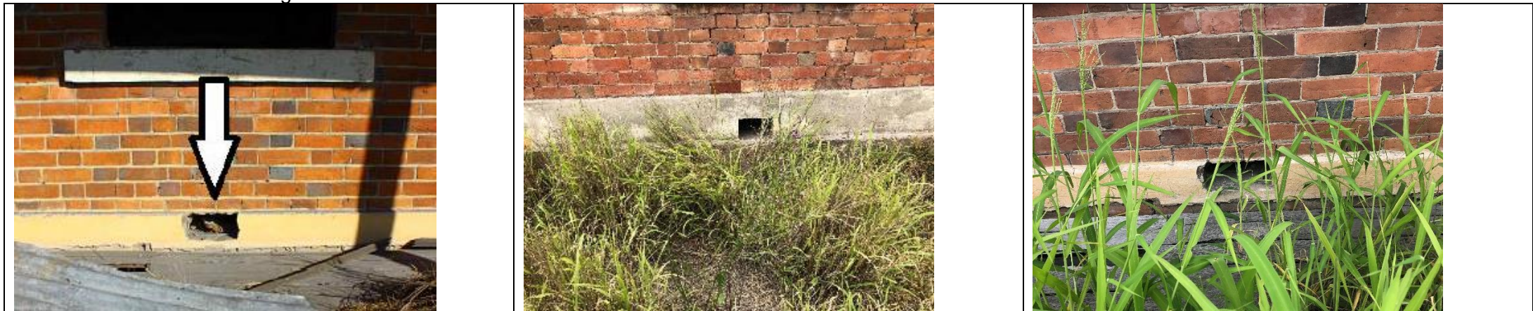
View of ventilation grilles
