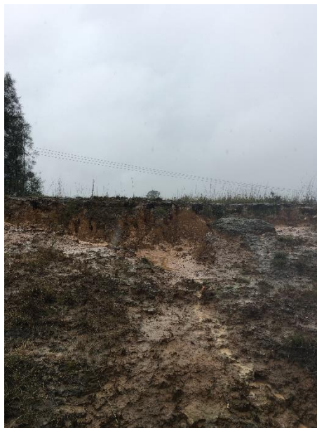
Plate 9 Erosion (top of right bank)
