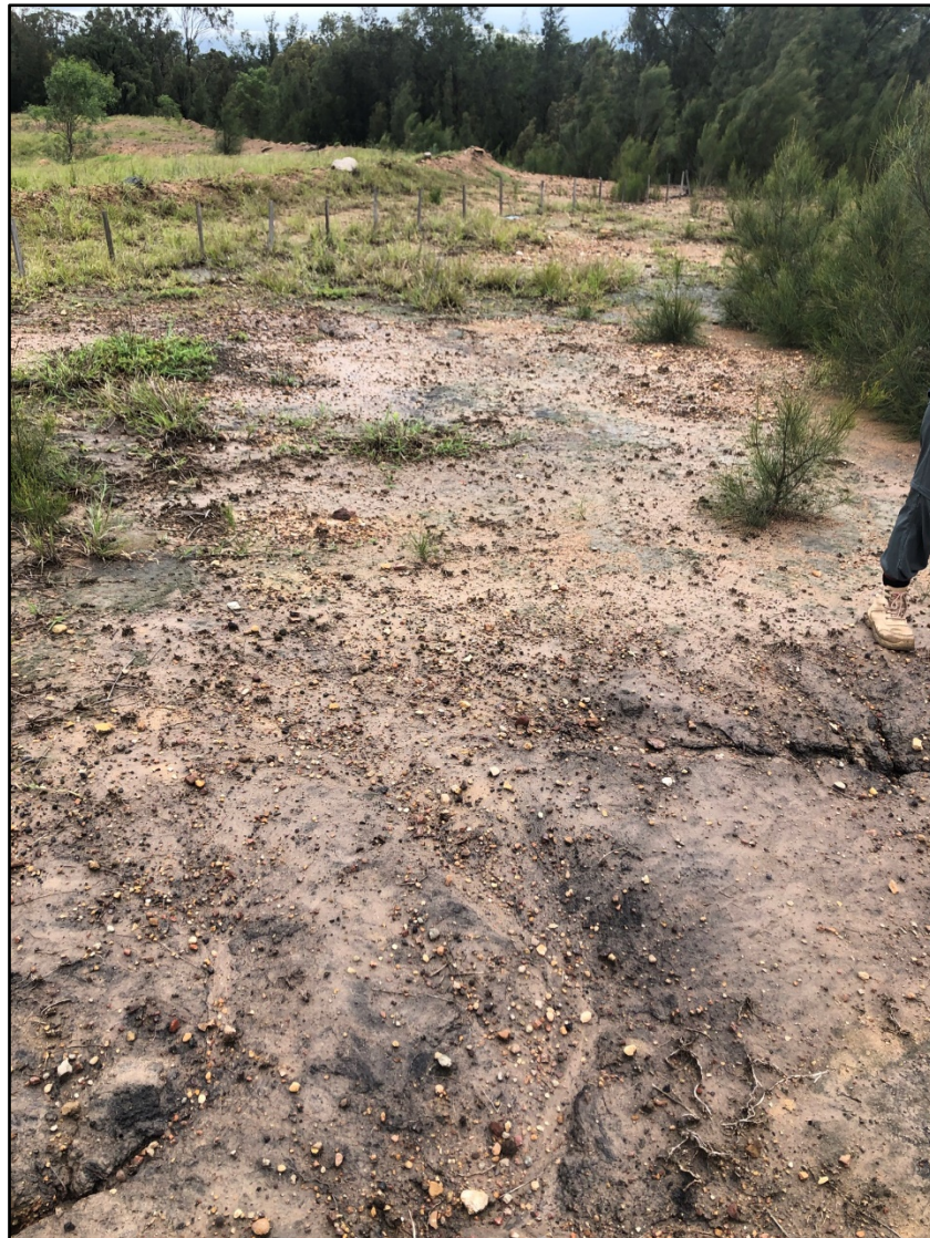
Sheet wash erosion at MTW-548
