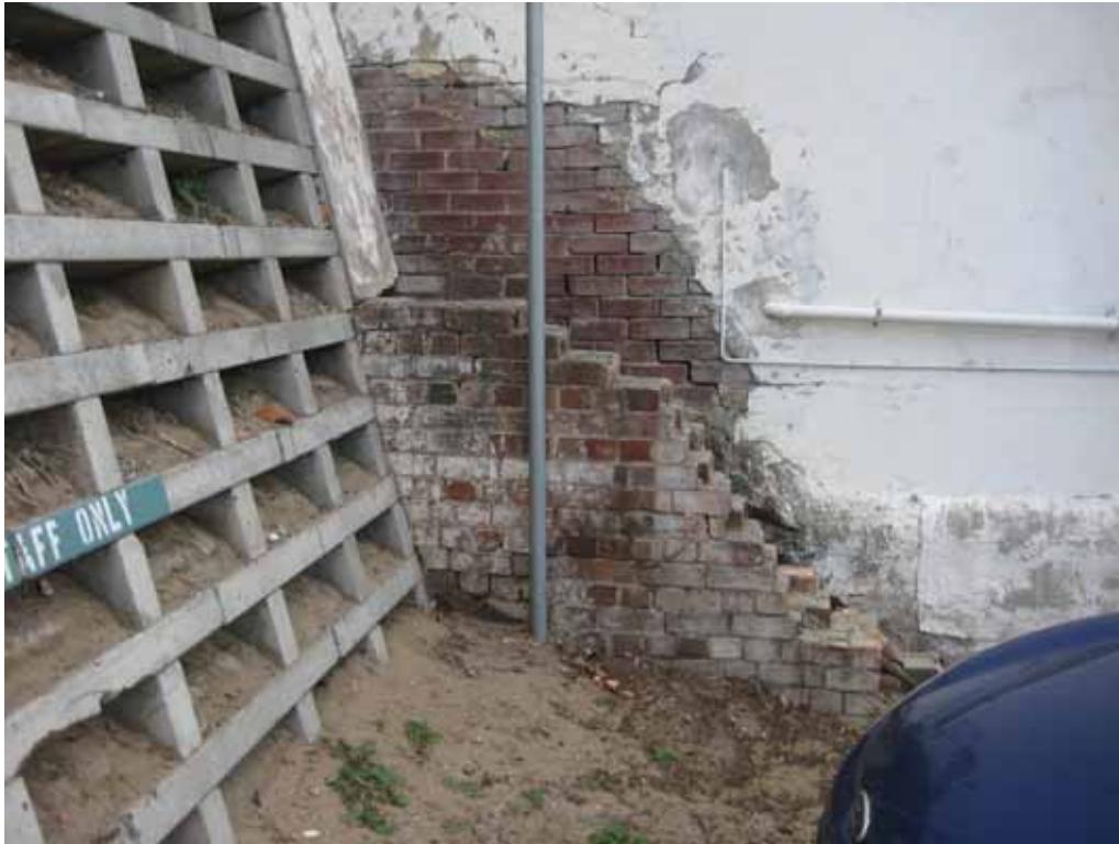
Figure 54. South-west portion of Gibson Street car park, showing intrusive crib-lock retaining wall at left and wall of 15 Gibson Street (Gibson Street Gallery), in front of which are the ruinous remains of the western wall of Devon Terrace, the bricks of which appear to bear the frog 'BOWTELL'. EJE
