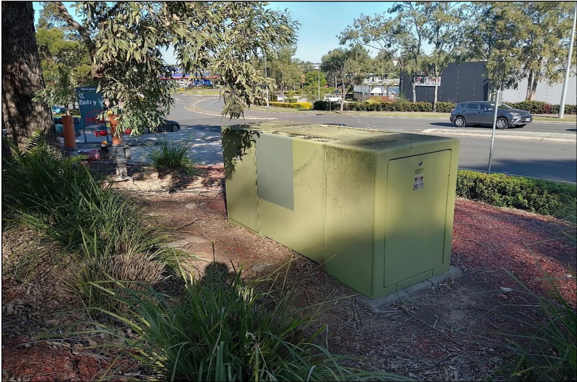
Photograph 11 - Pad-mounted transformer identified west of the boundary.
