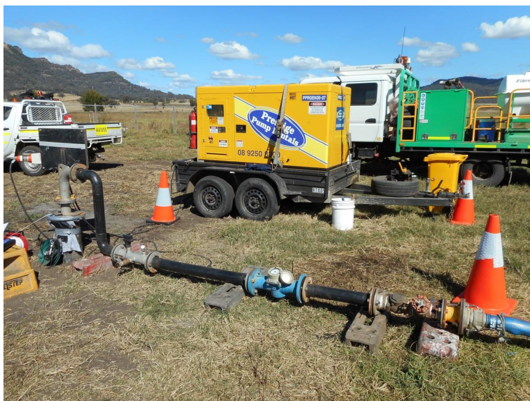
Figure 4-10 Headworks and flow meter setup
