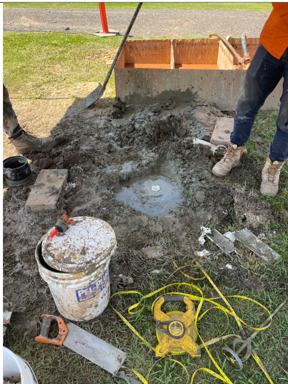
IMAGE 8 – Quickset concrete installation prior to addition of gatic cover on installed piezometers.
