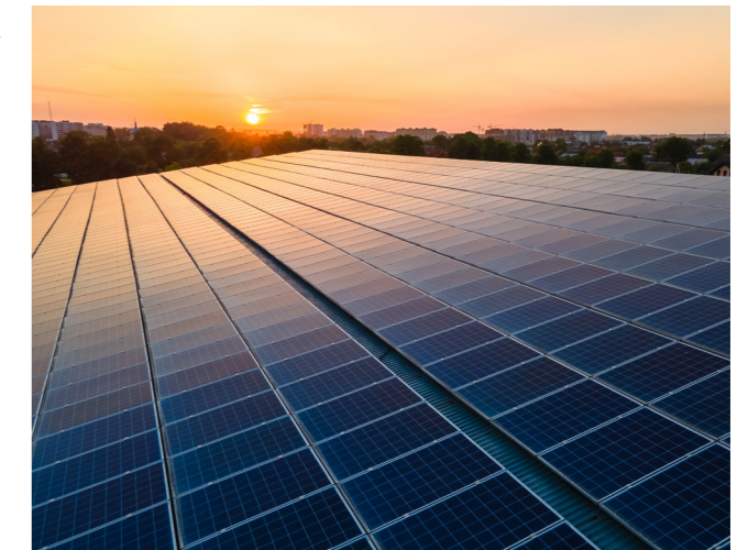
Provide PV panels for renewable energy
