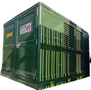
Kiosk substation image
