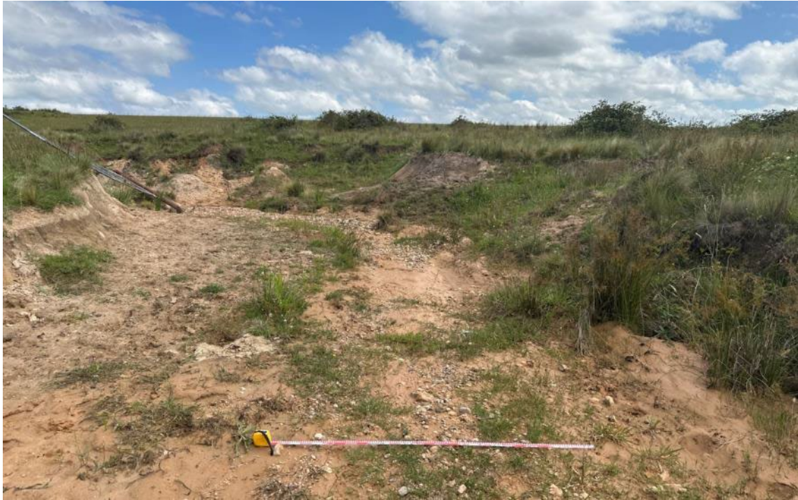
Figure 7.8 Exposures from water erosion in the eastern portion of SU2.
