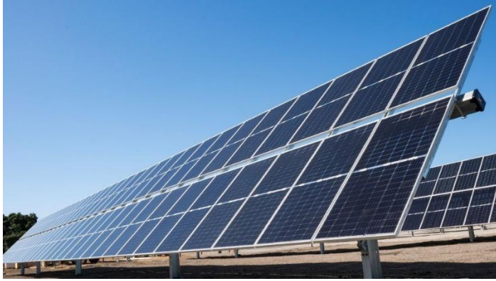
Figure 3 Typical photovoltaic module layout in 2P configuration
