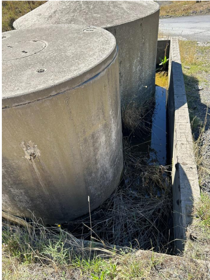
Photo 25: Septic tanks showing minor water accumulation in bund.
