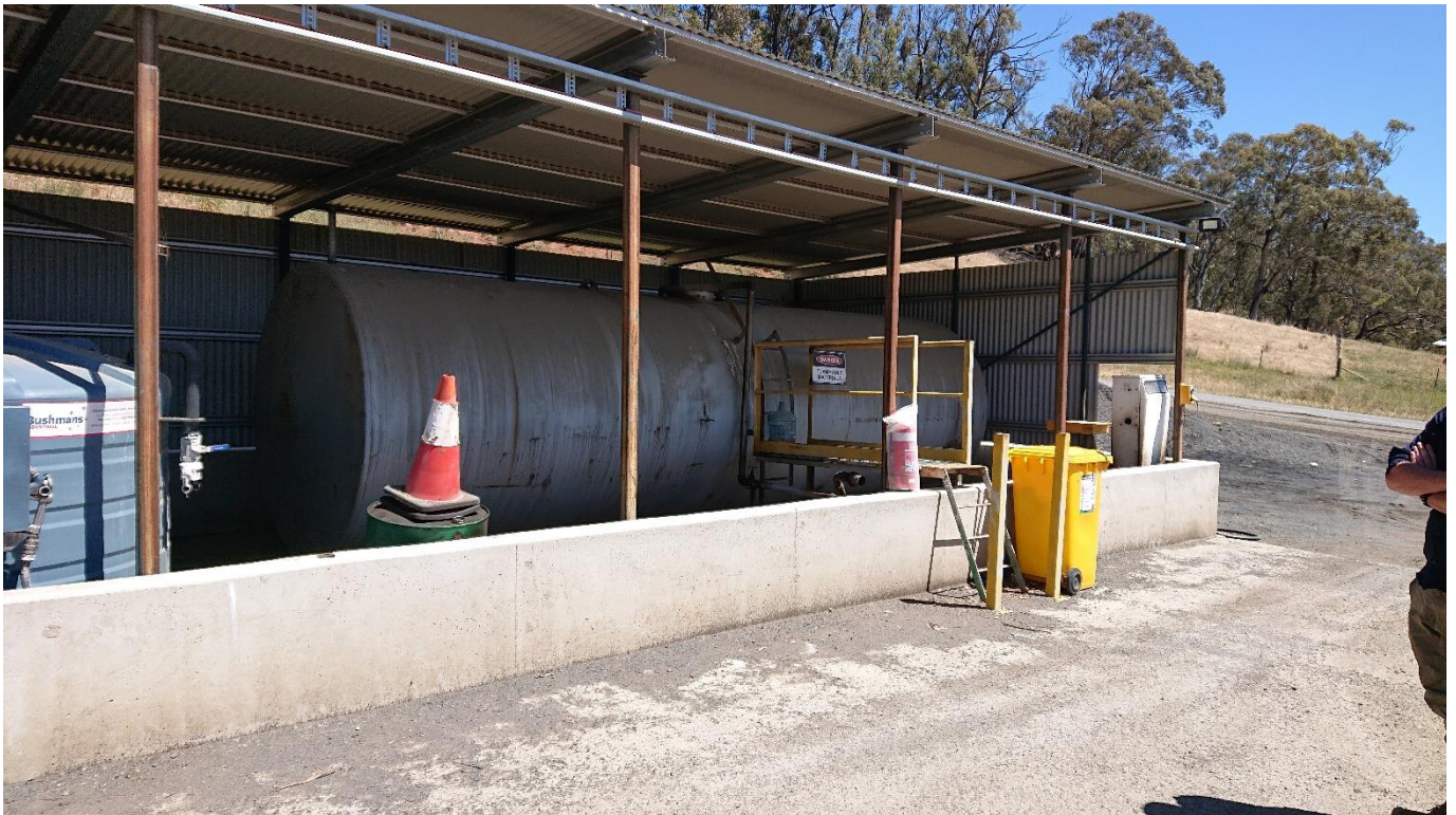
Photo # 4 - Diesel Fuel Storage
