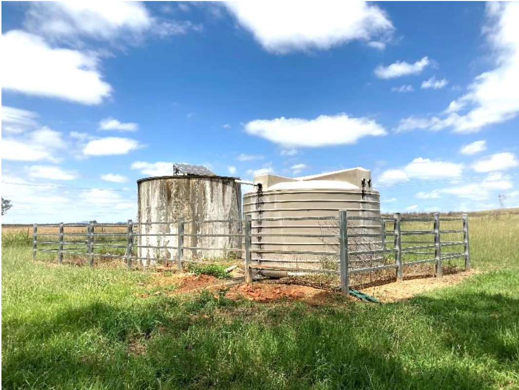
Figure 3-6: Existing groundwater bore (GW055998) – located at the southeast boundary of the Project Site
