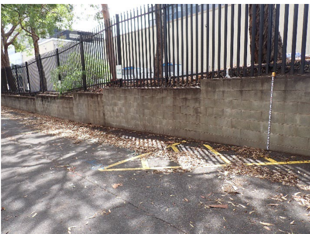
Figure 29 – Difference in level relative to adjacent property at 5 Thomas Hold Drive.
