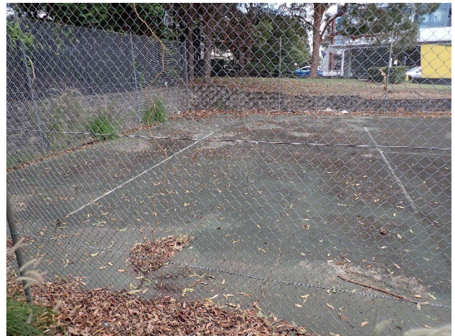
Figure 26 – Tennis court on north-western boundary, view north-west. Note how the level surface has been cut into the sloped terrain.
