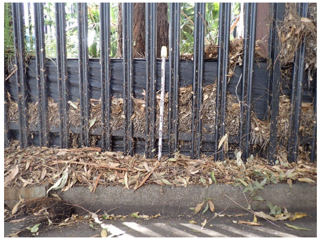
Figure 22 – Difference in level relative to adjacent property at 5 Thomas Hold Drive.
