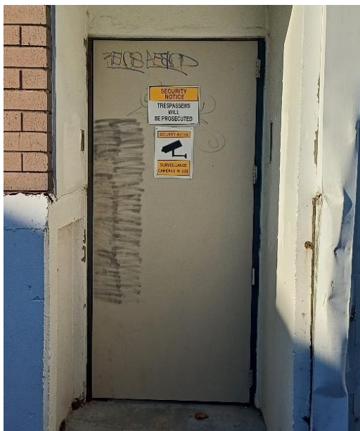
Figure 13 Signage indicated security measures and evidence of vandalism (graffiti), Wyndham Lane
