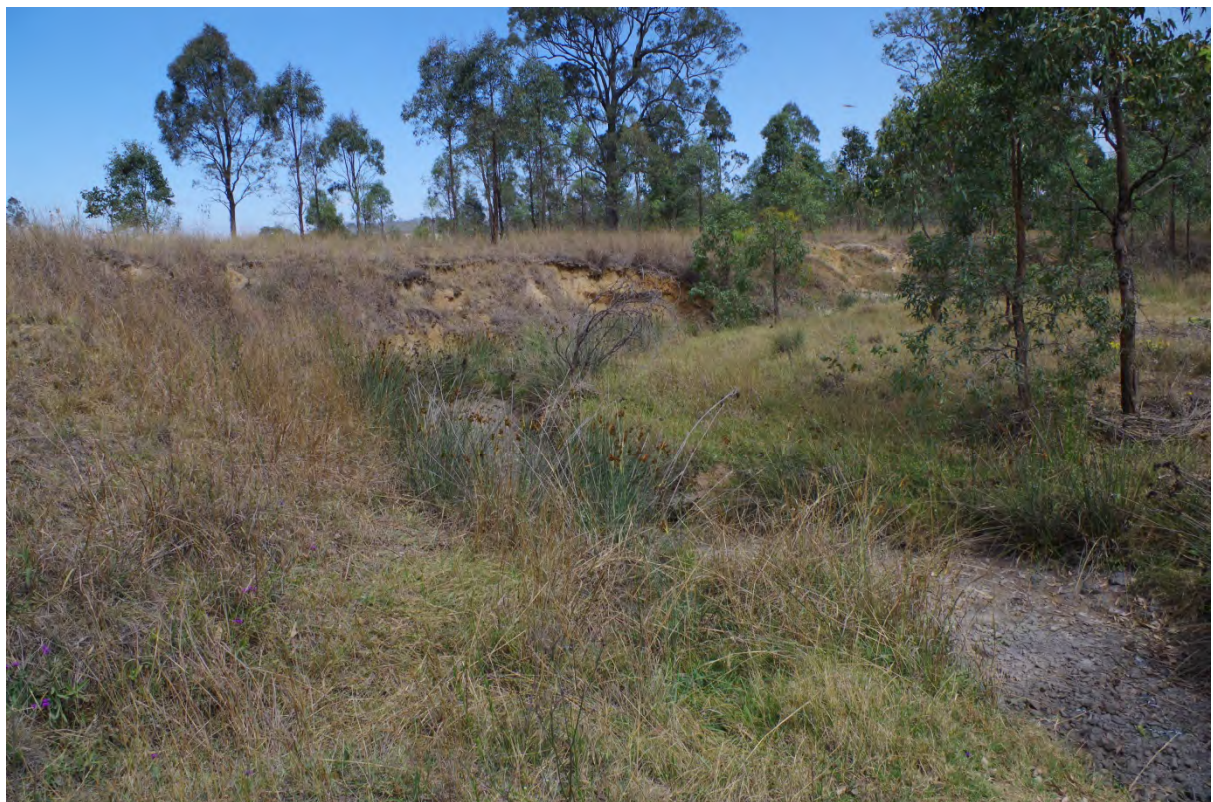
Chainage 10419 Looking Downstream. Undercutting on Left Bank
