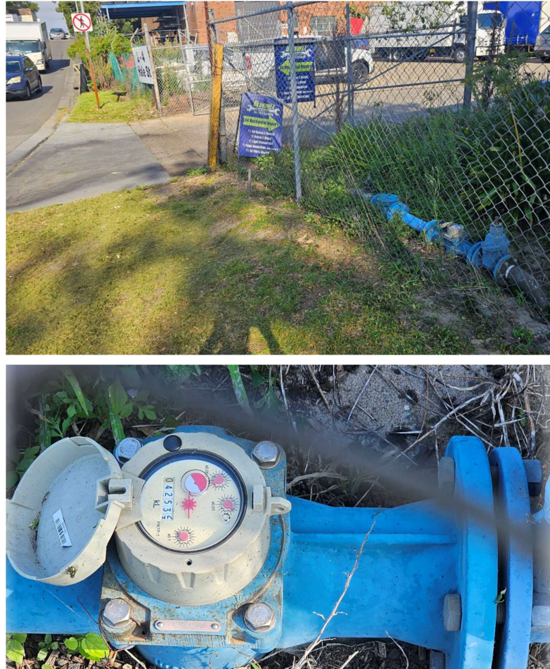
Figure 5 - Existing Water Meter
